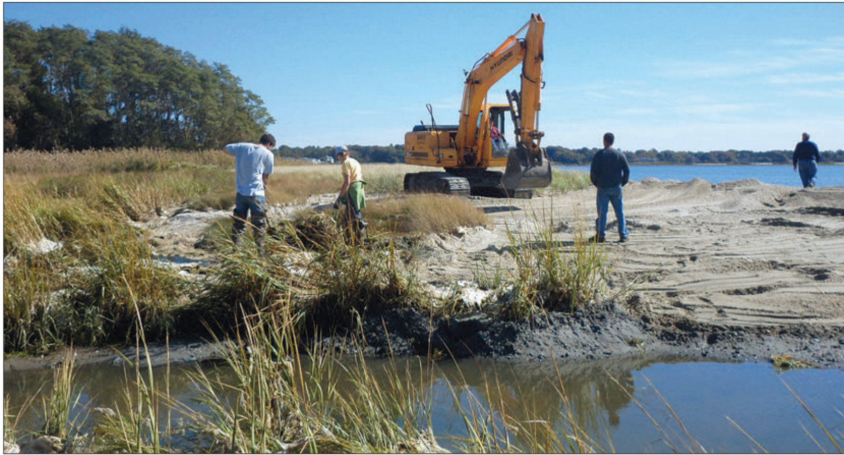
Workers used backhoes and other equipment to clear the creeks leading to the salt marshes at RISD beach recently.
