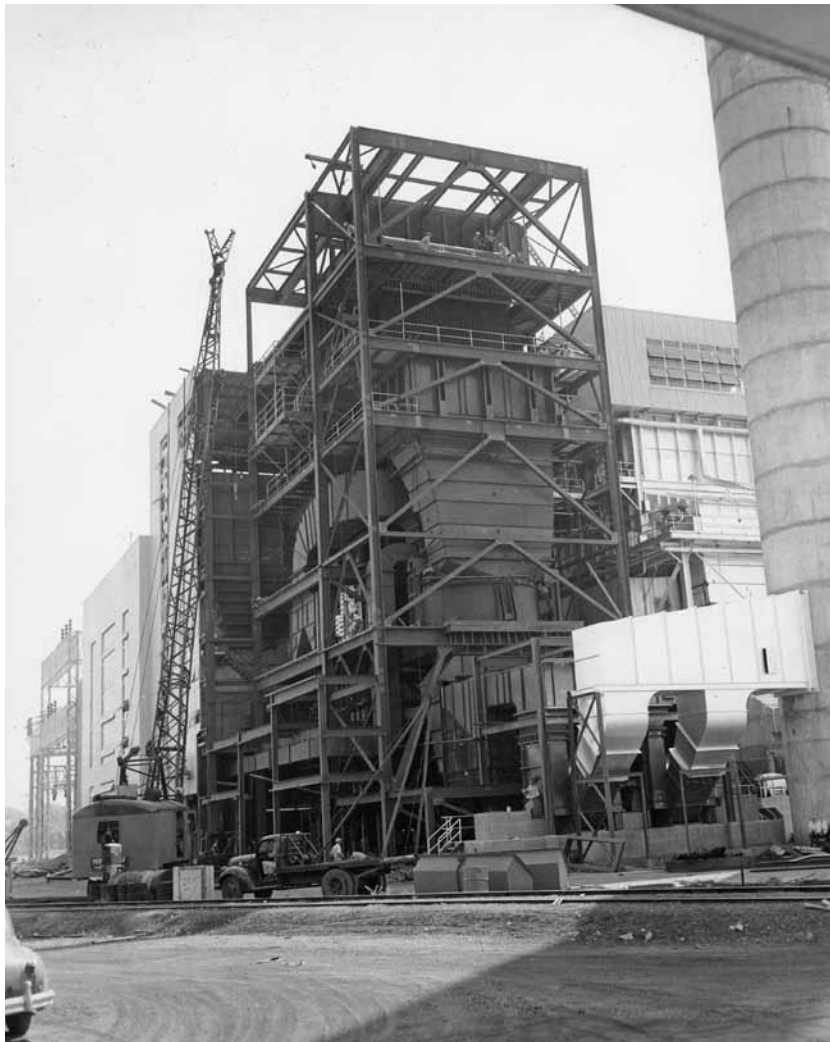
LEFT: Northwest elevation at Riverton, showing the progress of the boiler construction, August 24, 1953.
