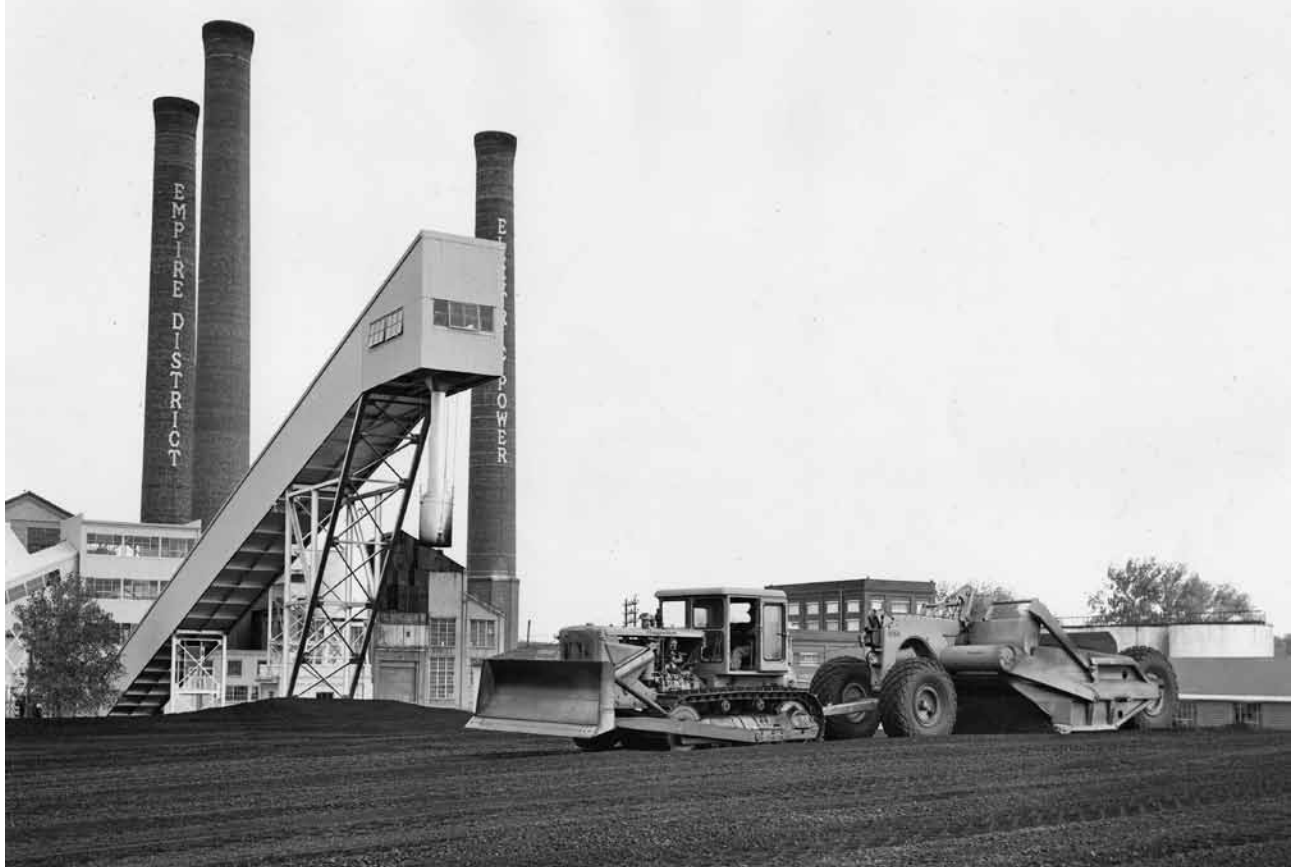
ABOVE: Caterpillar Diesel D8 tractor equipped with No. 88 Bulldozer and No. 80 Scraper, November 4, 1953, at Riverton.
