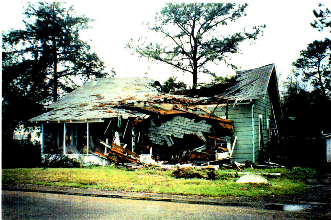
Figure 4-4. Residence Destroyed by Tree -- Opp, Alabama
