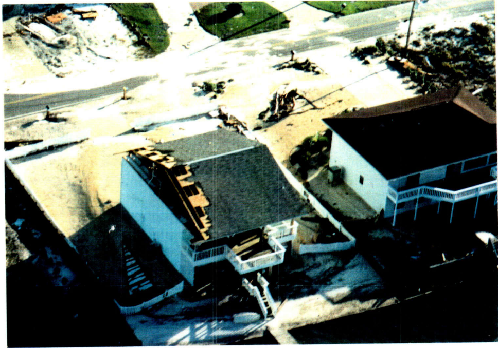
Figure 4-1. Roof Failure -- Holiday Isle, Florida
