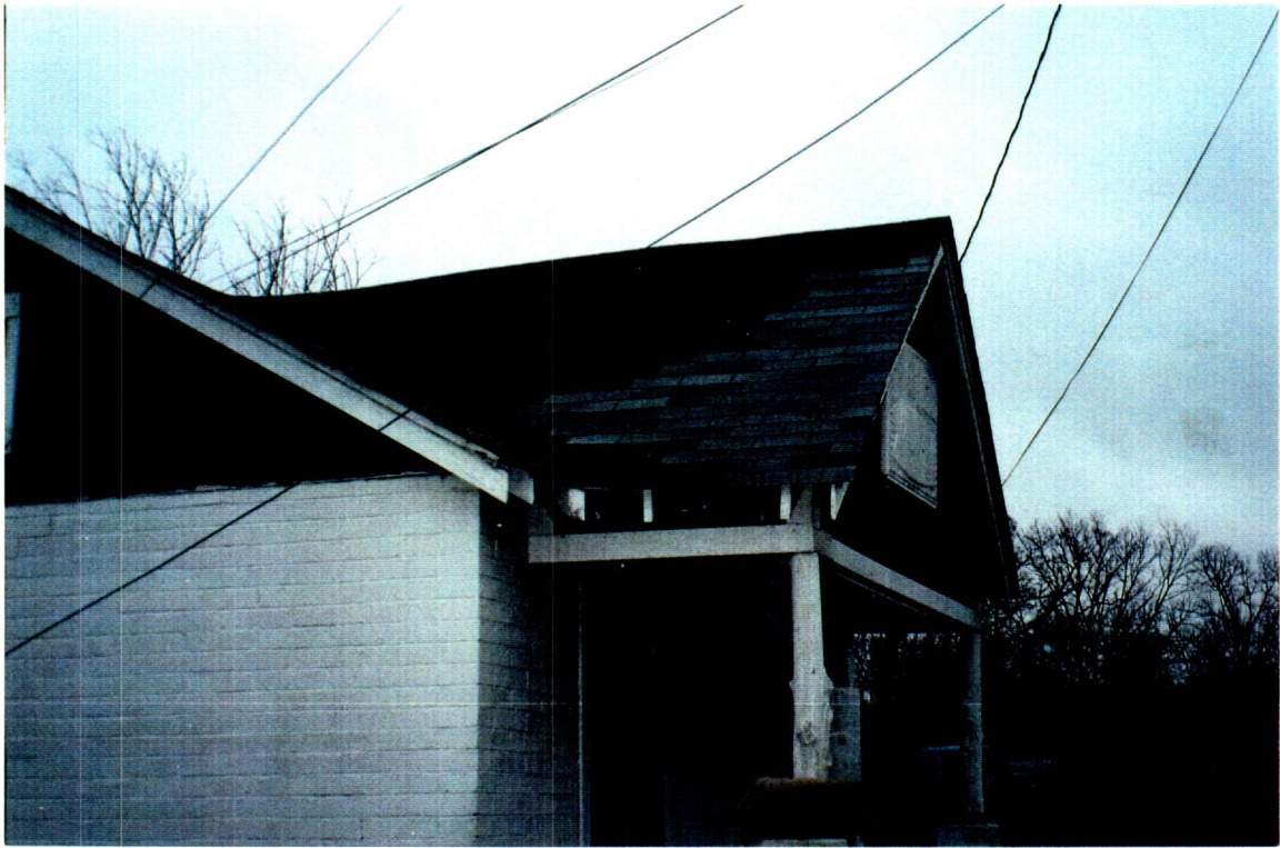
Figure 4-5. Roof Covering Damage -- Opp, Alabama
