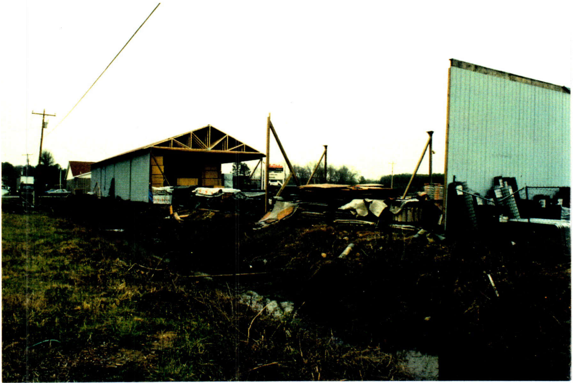
Figure 4-9. Wind Damage to Warehouse -- Walker County, Georgia
