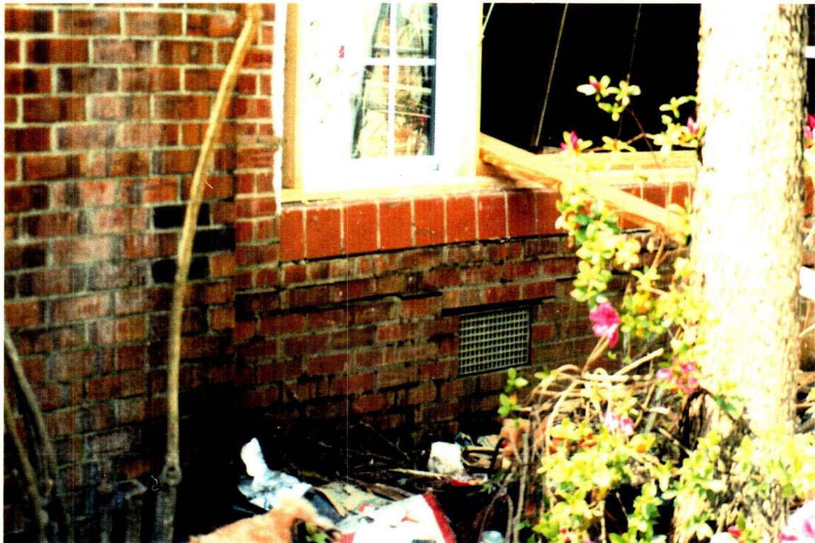
Figure 4-3. Residence Damaged by Tree -- Okaloosa County, Florida
