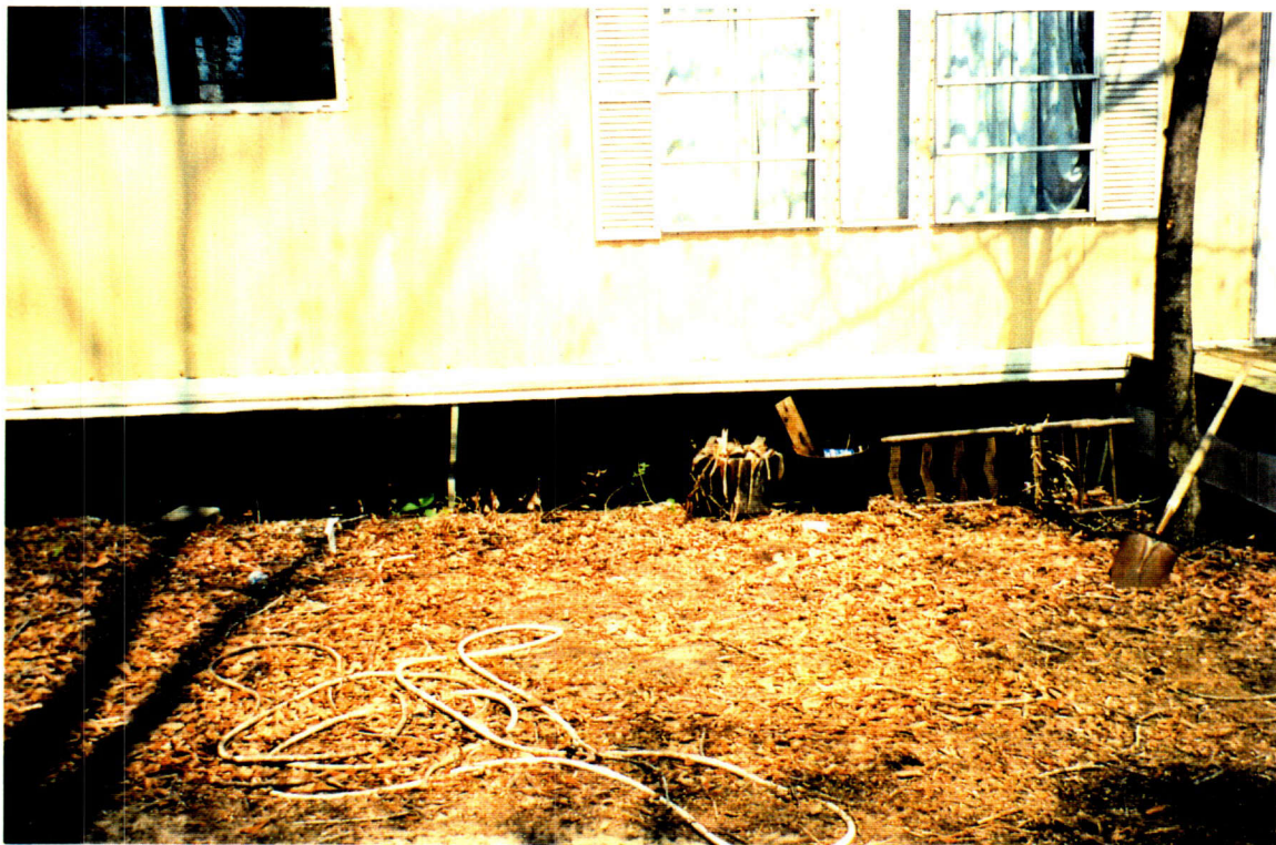
Figure 4-6. Manufactured Home Shifted by Wind
