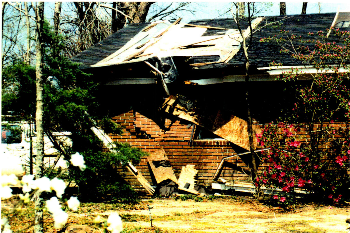
Figure 4-2. Residence Damaged by Tree -- Okaloosa County, Florida
