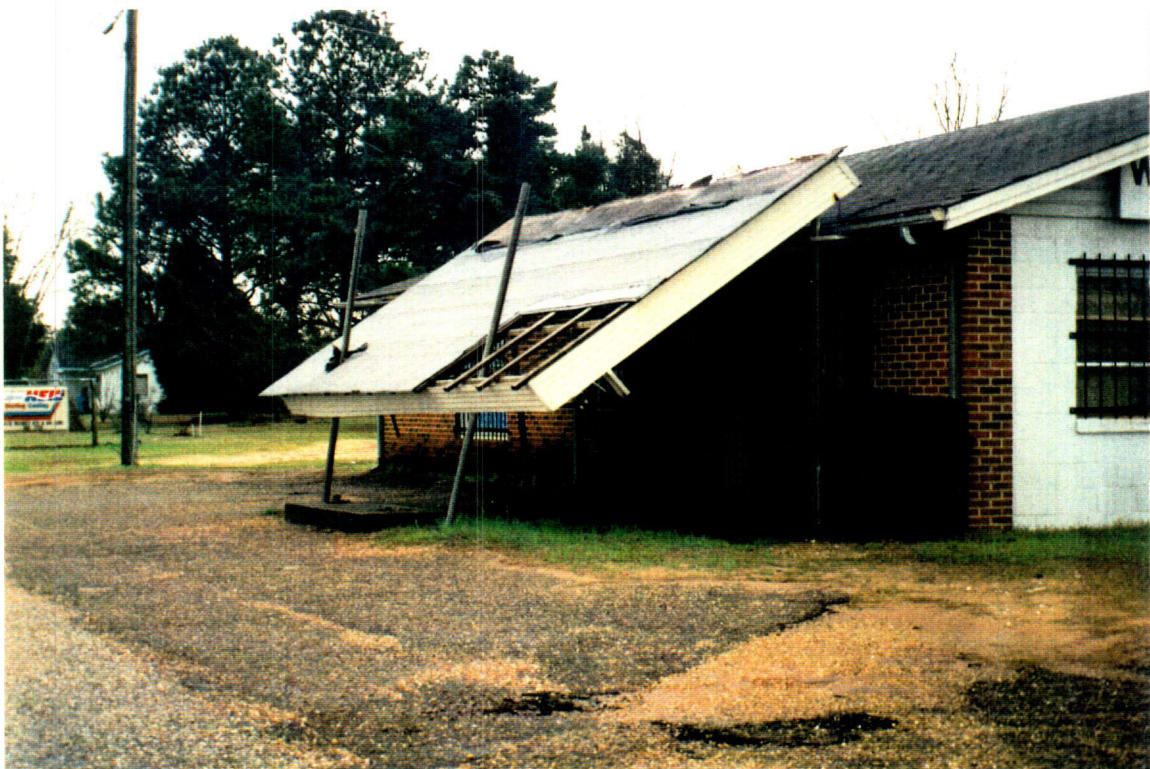
Figure 4-8. Roof Canopy Damaged -- Troy, Alabama
