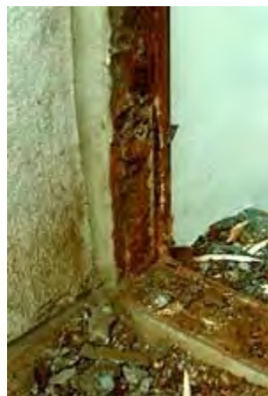
A severely deteriorated frame, such as this, can be replaced in kind. Photo:
