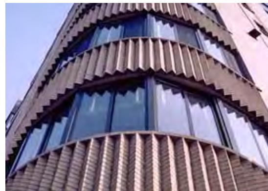
The historic steel sash (see photo above) was removed and replaced with modern aluminum sash, resulting in a negative visual impact on the building's historic character. Photo: NPS files.
