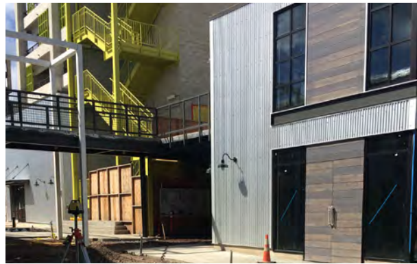
The new Salt Building Project by Kamehameha Schools Image from VIA Architecture
