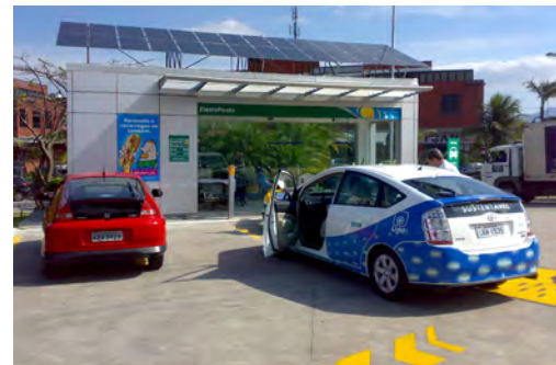
Solar powered charging station in Rio De Janeiro Image from Andricos
