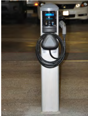
The City of Honolulu installed public EV charging stations include one in at the Neil Blaisdell Center. Image from City of Honolulu
