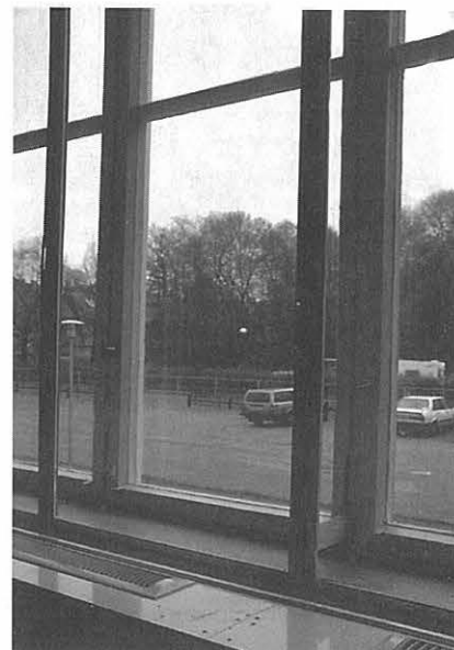
Steel frame detailing of meeting room windows. Photo: T. Almqvist.
