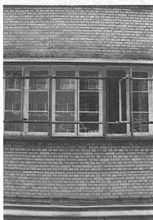
Employment centre. Window in the south facade of the administration wing. Original steel windows with single glazing and casement windows. In the background the timber windows added after 1935, that will be removed as part of the restoration.
