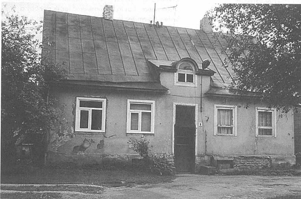
A simple house of the 1920s by Herbert Johanson now displays a doubtful demonstration of progress. The PVC units to the left contrast sharply with the old wooden windows to the right. All photos: Andri Ksenofontov.
