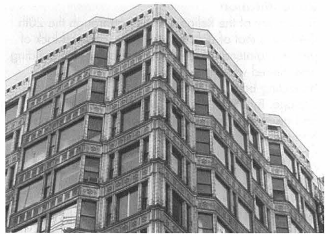
Reliance Building cornice before restoration, 1994. Photo: T. Gunny Harboe.
