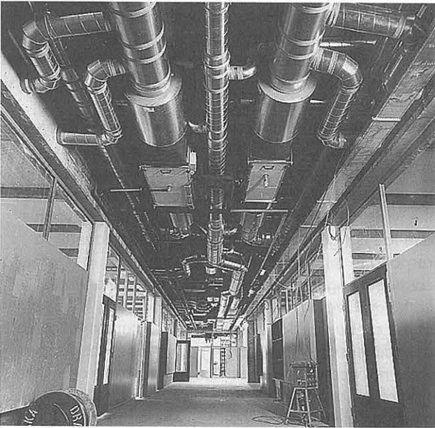
The amount of services packed between the lateral girders, before the vertical louvre ceiling was installed. Photo: Hans Vroege.
