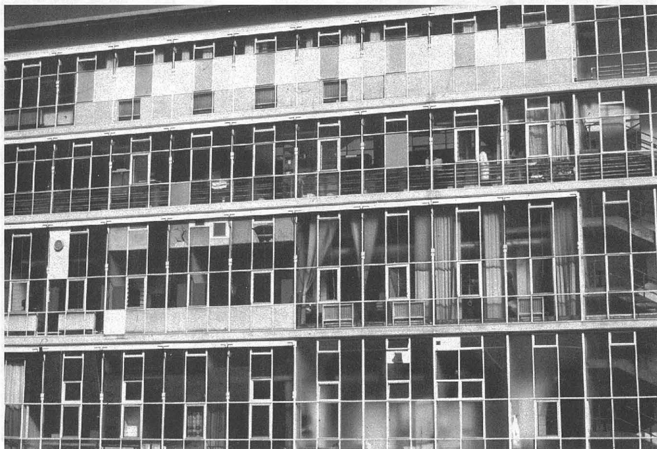
The Boots building before repairs were carried out, showing the original glazing and replacement hardboard, louvres, extract fans and blank panels.
