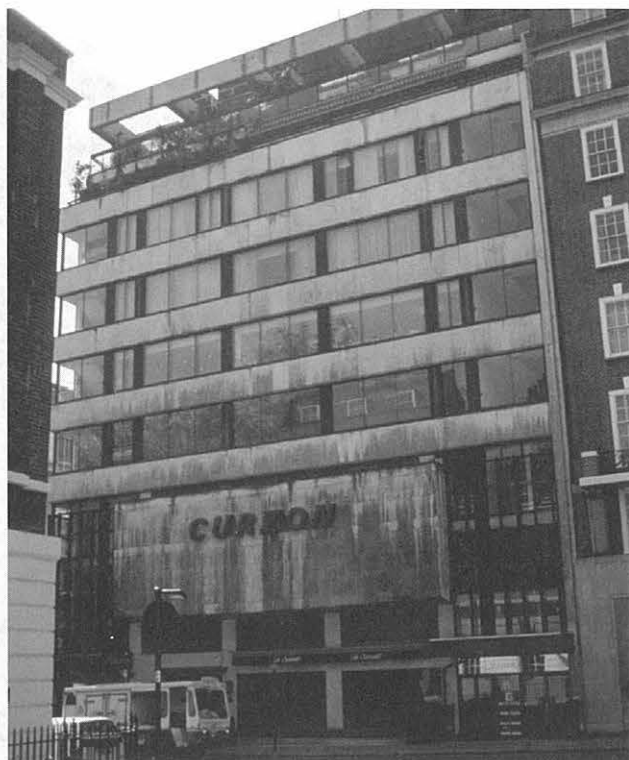
The Curzon Cinema, Central London, where the proposal to replace the aluminium framed secondary glazing with a tilt and turn PVC system, would have severely damaged the appearance of this listed building and meant the loss of a rare survival of a pioneering glazing system from the early 1960s.
