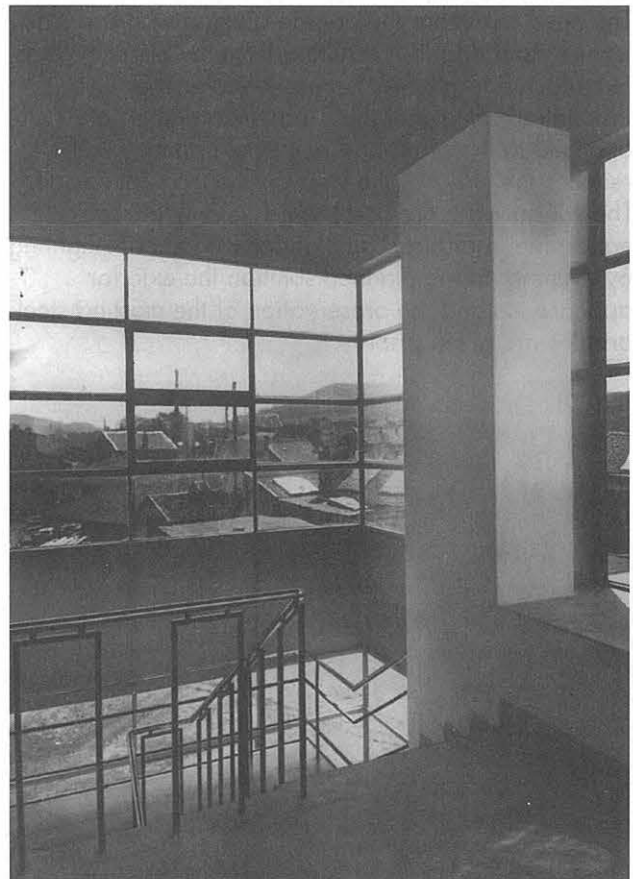
Interior view of the staircase (second building phase) of the Fagus factory in Alfeld with single glazing, even after the restoration.
