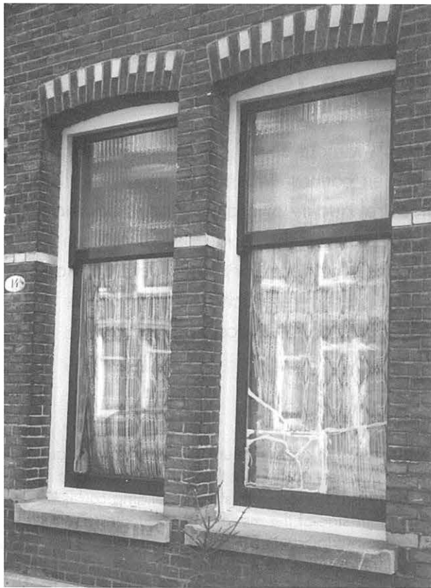
Detail of a 1900-1920s timber window with stationary top light and recessed sash.
