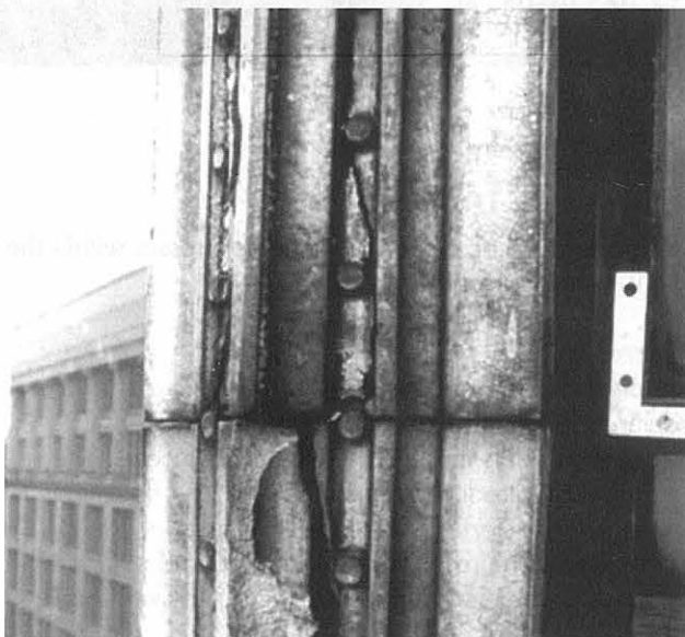
Deteriorated terra cotta mullion piece, 1994. Photo: T. Gunny Harboe.
