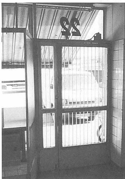
Entrance door showing lower and upper vents to dry shops at night.
