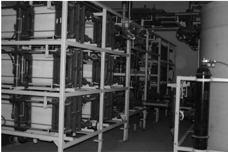
Figure 48: Part of the 500 kW, 1000 kWh Prudent Energy installation for China Grid, 2011
