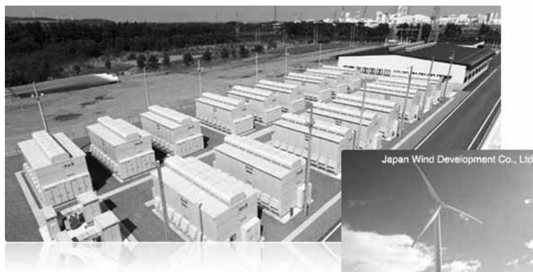
Figure 43: 34MW NaS battery operating at a 51MW wind farm in Japan 132
