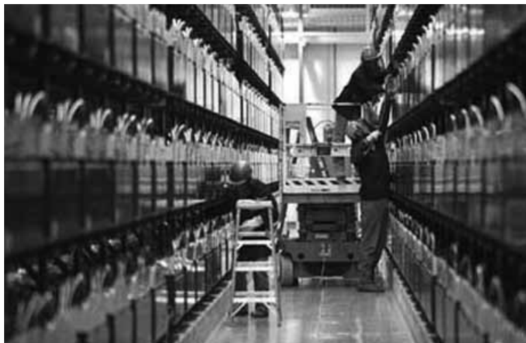
Figure 46: 40MW, 15 minute nickel cadmium battery, Golden Valley, Alaska (1992) 137
