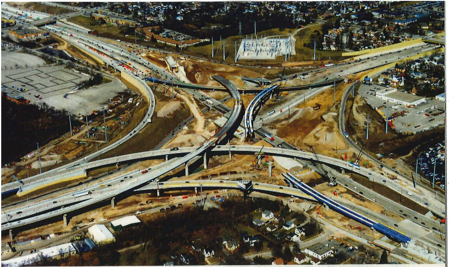
The Zoo Interchange project is the largest in Wisconsin at $1.7 billion, and bears the state's most complex work zone.
