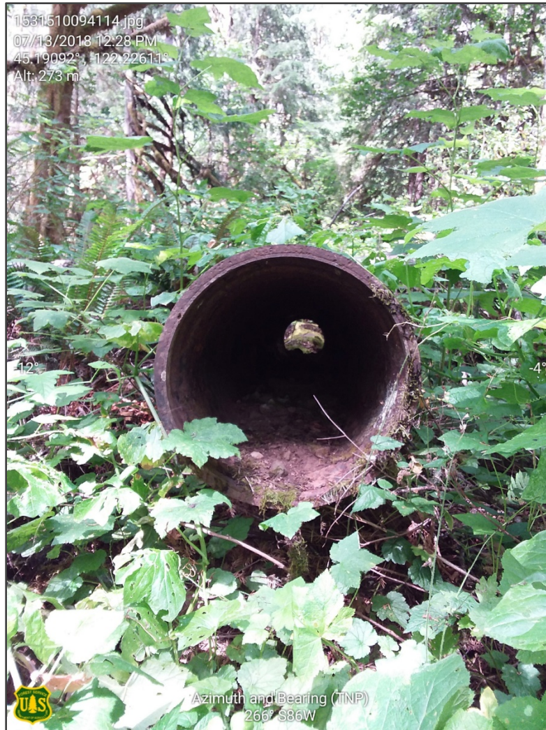
Figure 18. Part of the South Fork Water Board Pipeline
