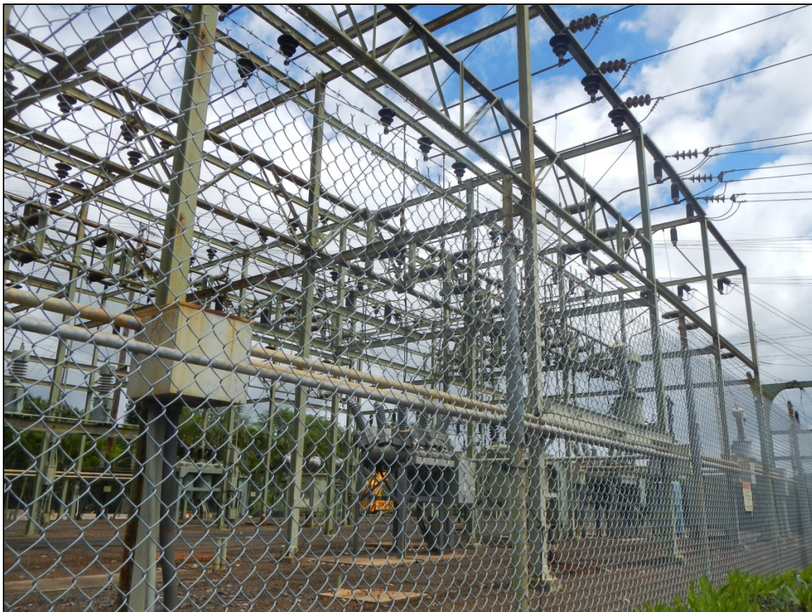
Figure 3.14 Photograph of Existing 46 kV Substation
