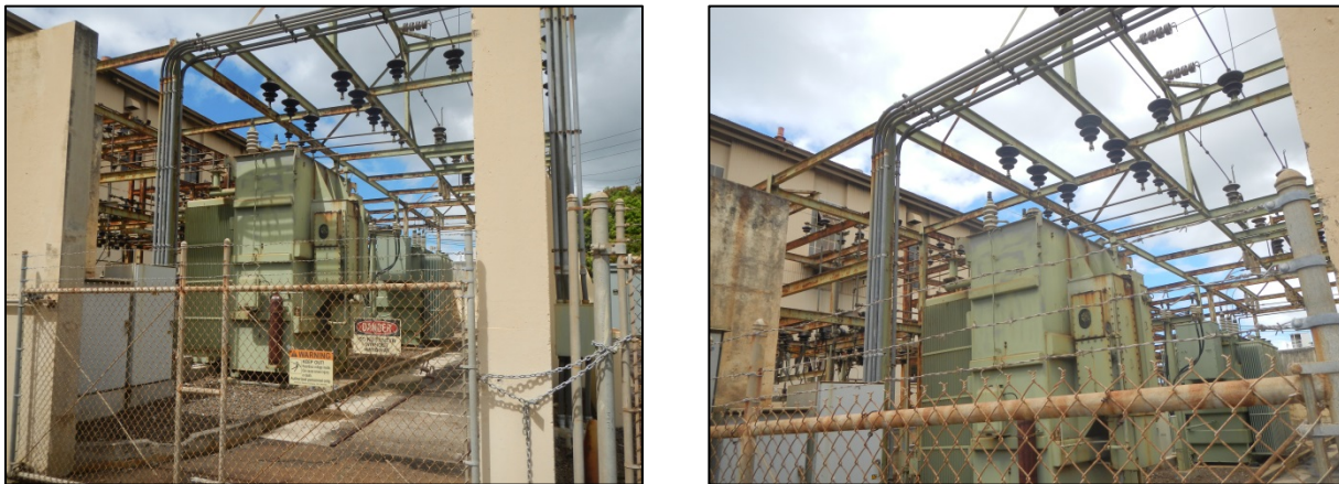
Figure 3.11 12 kV Substation at WGS to be Demolished
