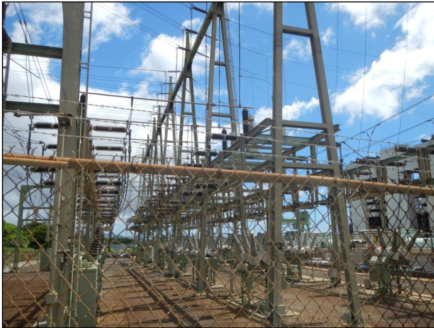
Figure 3.12 Photograph of Existing 138kV Substation
