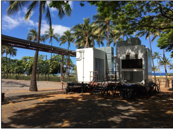
Figure 3.9 Photographs of Typical VFD Units
