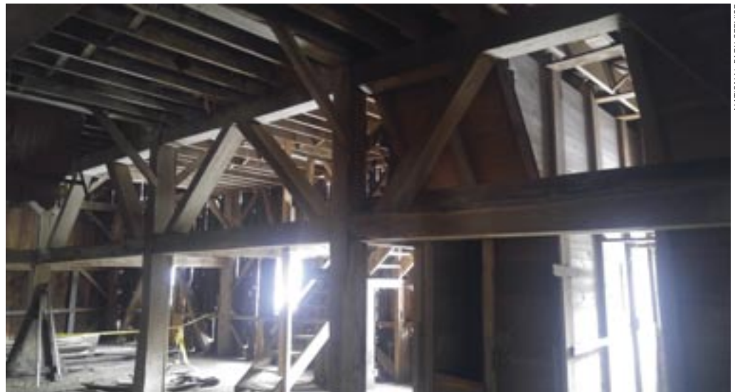
Right, the truss system on the barn's second floor was built to support and store a steam engine and other apparatus.
