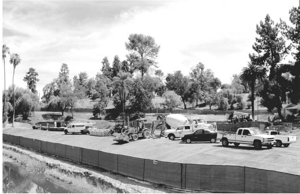
HILLCREST IN FULL SWING Construction of the front bridge and other improvements at Hillcrest on Harbor is really picking up steam now, as you can see from this view, taken last week.
