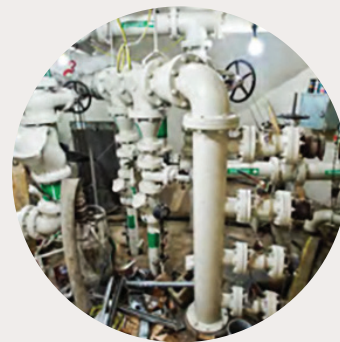
Pump rooms (ROW)
