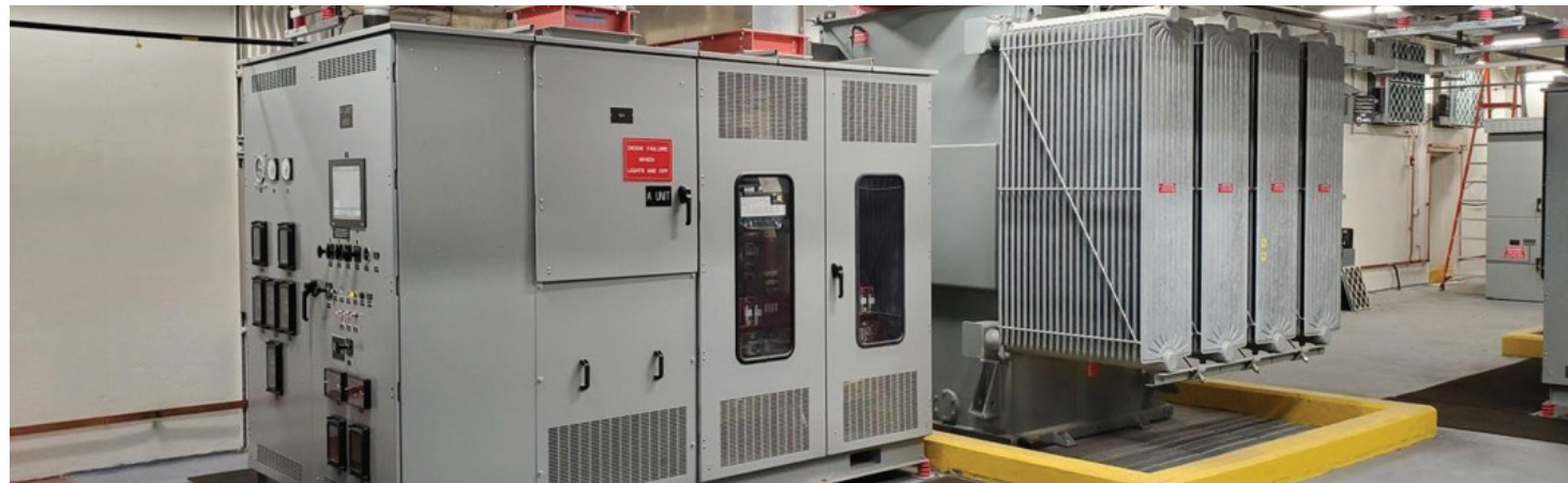
Maspeth Substation, NYCT
