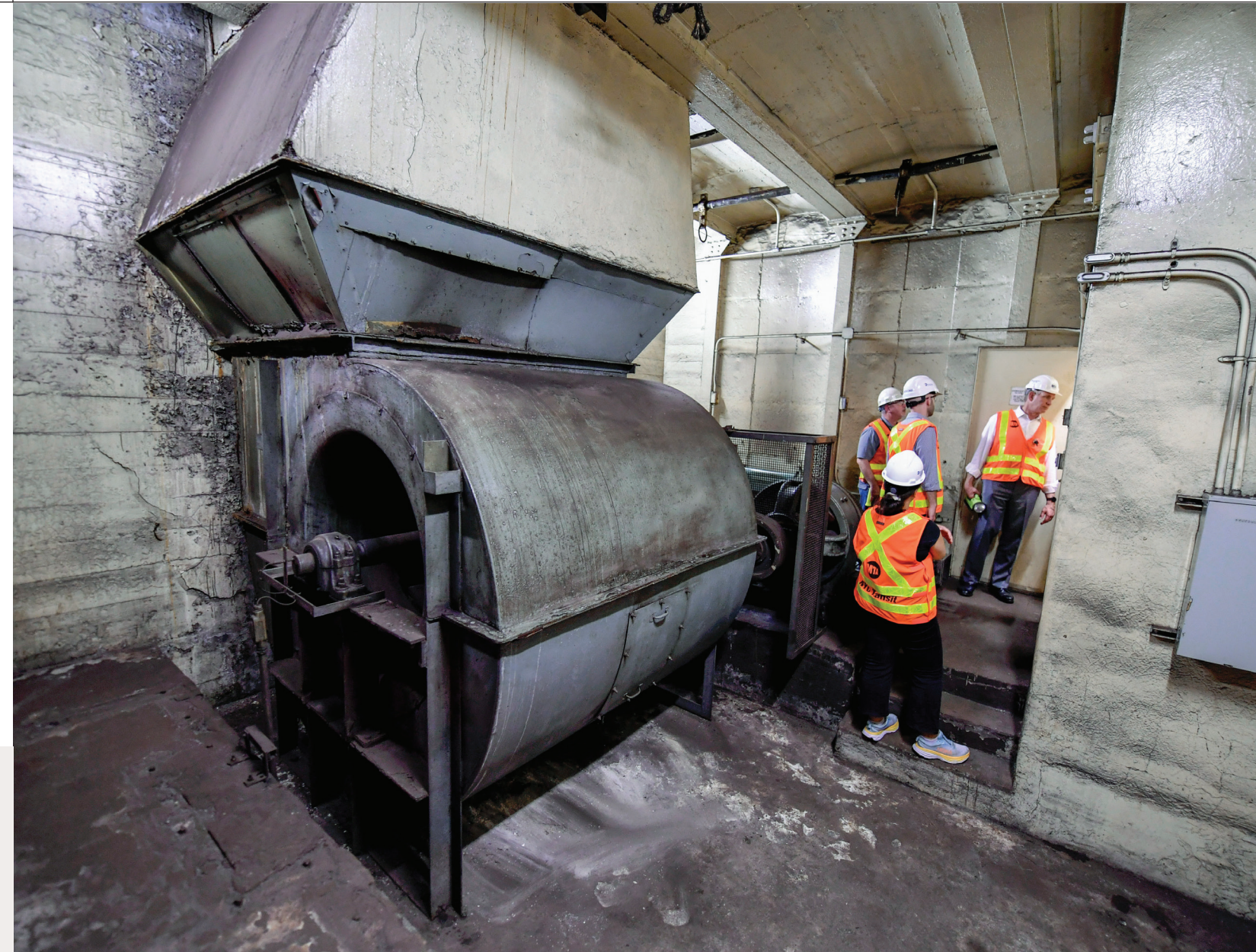
Prince Street Fan Plant
