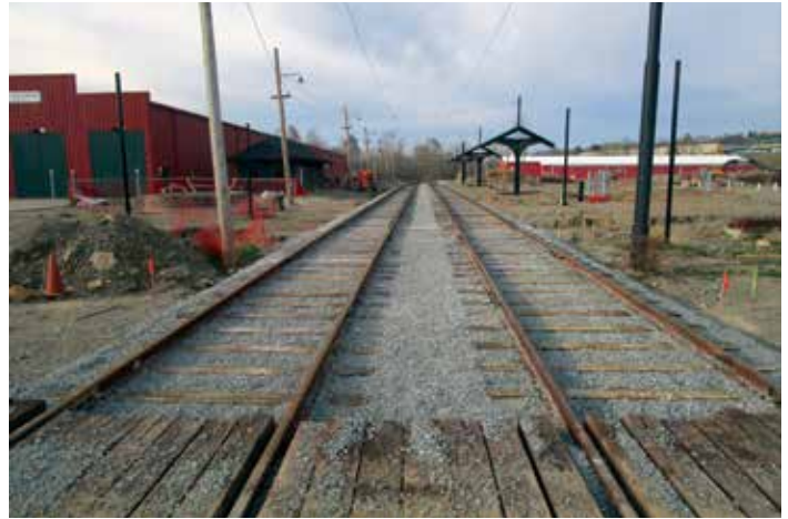
As part of the Pennsylvania Trolley Museum's larger East Site project, the double track and overhead wire portion of Trolley Street is complete and operational. Brick paving will be installed during 2022. Visible in the distance is the Artifact Preservation Building. Last summer a wye was completed permitting the last two streetcars to enter the building, so the entire 50-car collection is under roof for the first time.
