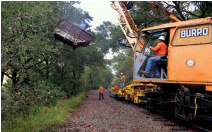
Steve Barkkarie lifting box loaded with junk with the Burro Crane while Doug Vanderlee is ready to guide the box into place on the heavy hauler.
