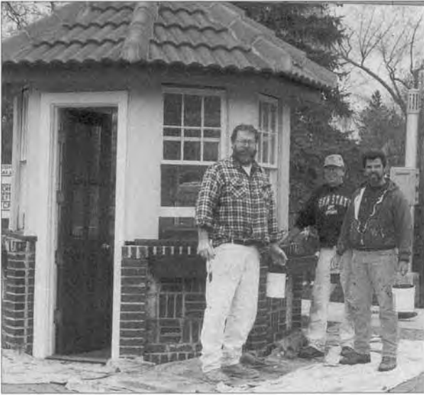
One of Hillsdale's central figures, the police booth, gets a face lift for Hillsdale's 100th Birthday. Rick Winkler, Stewart Blank and John Hering at work providing a fresh coat of paint.
