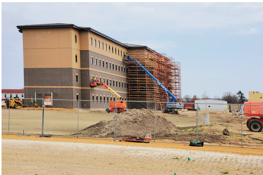
Construction of a new transient troop training barracks at Fort McCoy, Wisconsin, April 2021
