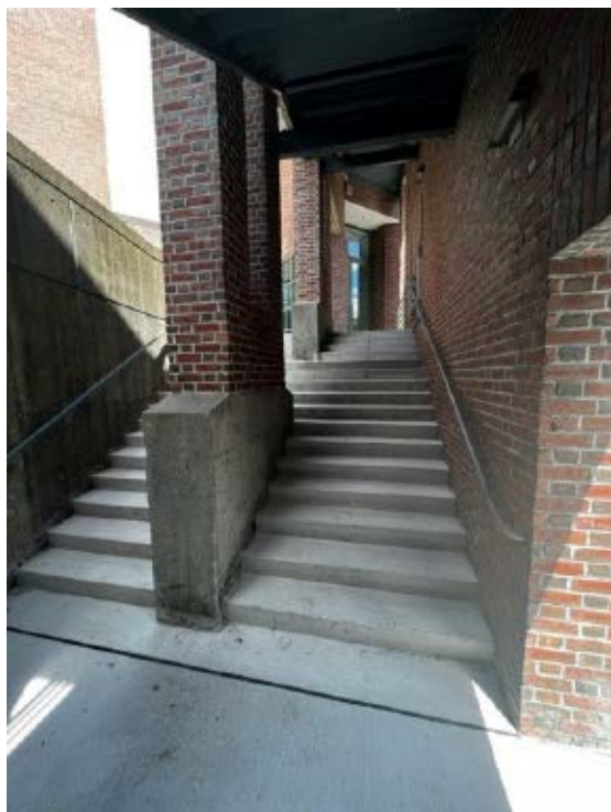
Nearly completed stairs leading to the museum's south entrance facing Lebanon Street, Hanover. Photo by Andrew Turner.
