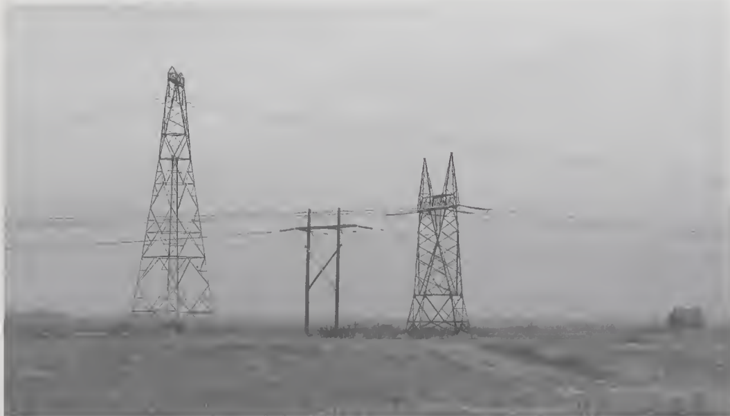
FIGURE 4. Intersection of three transmission lines north of the covered bridge on the High Marsh Road (Jolicure Road), Tantramar Marsh, New Brunswick, the site of numerous Common Eider collisions. Photo: A. Kennedy.
