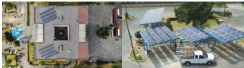
Fig. 2. SPV electricity generation system installed at CIC-IPN.
