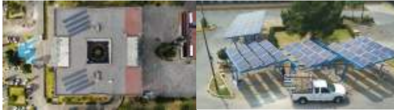
Fig. 1. SPV electricity generation plant installed at CIC-IPN.
