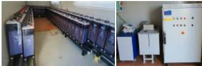
Fig. 3. Lead-acid batteries and DC/AC inverter.
