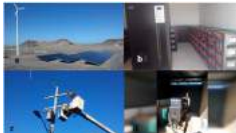
Fig. 2. Puertecitos, Baja California Power Generation System a), Inverter and battery bank b) Medium voltage power distribution system 13.3 kV c) and diesel electric generator d).
