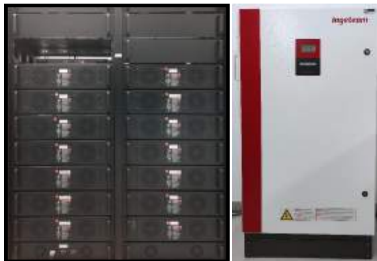
Fig. 4. LFP battery rack and inverter.
