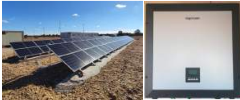
Fig. 2. Photovoltaic system (photovoltaic modules and DC/AC inverter).
