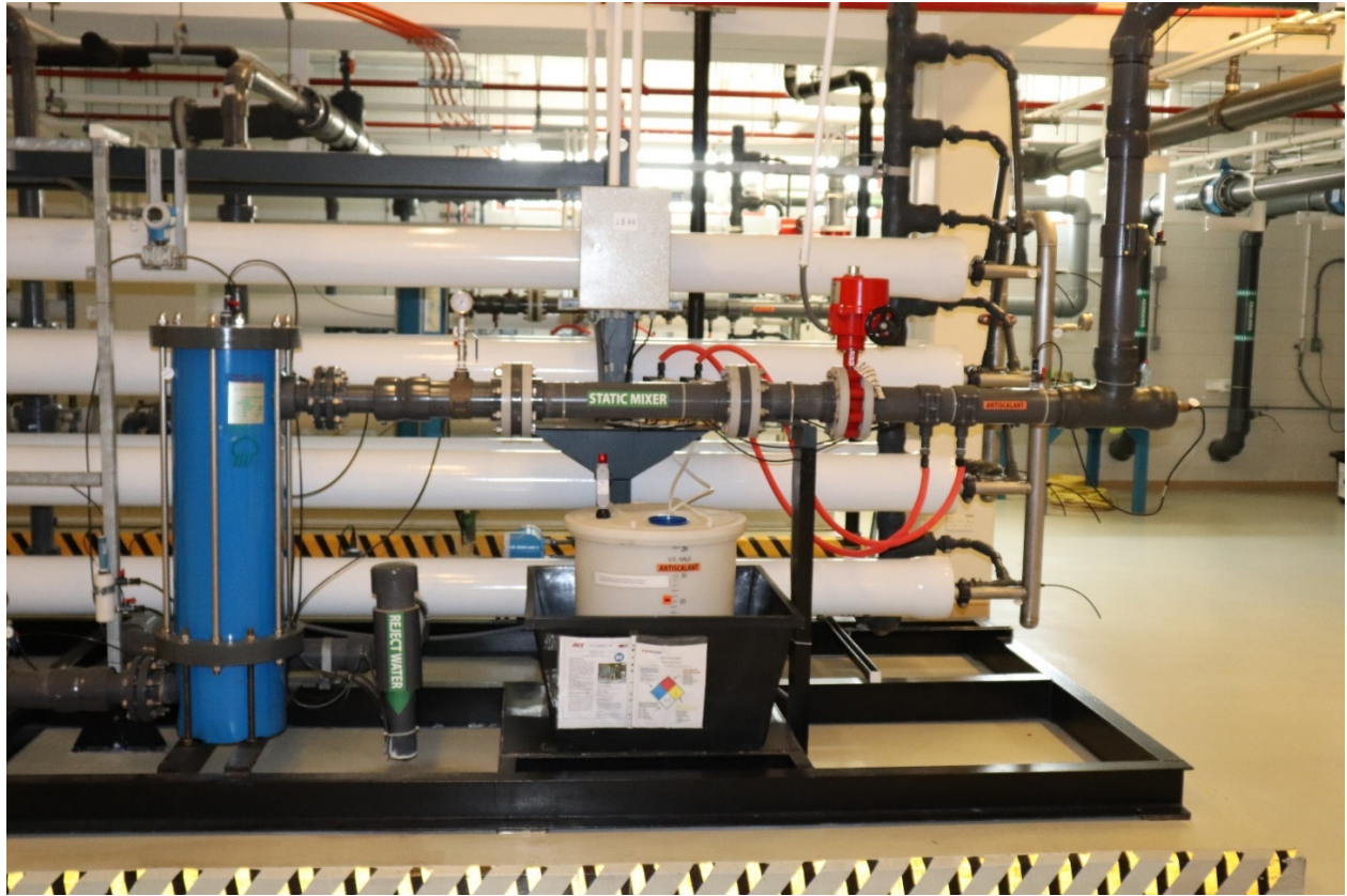
Figure 2 - RO Train 1, Right Front Side
