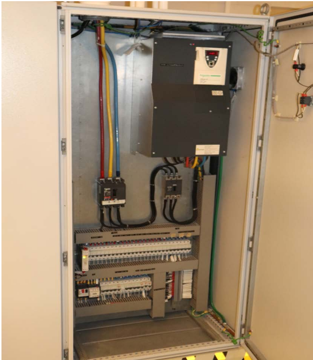
Figure 10 - Control Panel 2, Right Side, RO Feed Pump VFD, etc.
