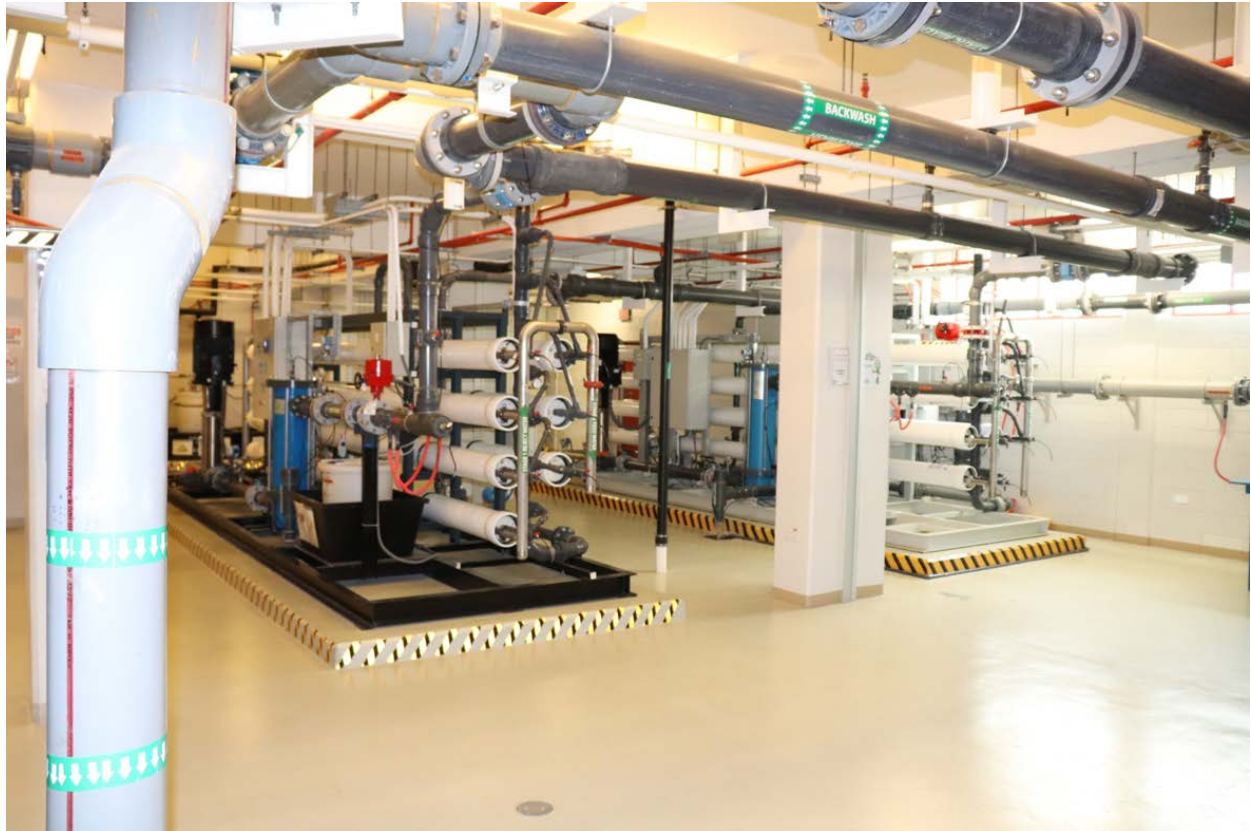
Figure 3 - RO Trains 1 and 2, Front Side
