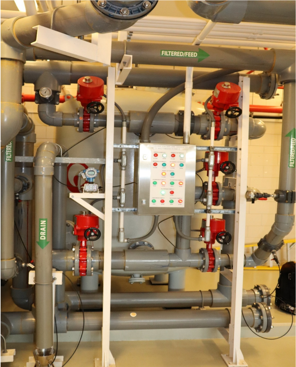
Figure 7 - Pressure Filter Unit 2 and Control Panel
