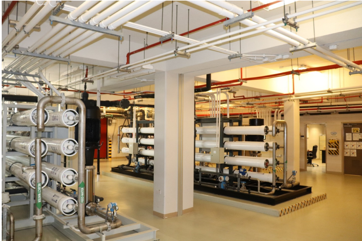
Figure 4 - RO Trains 1 and 2 (Rear Side of Train 1)
