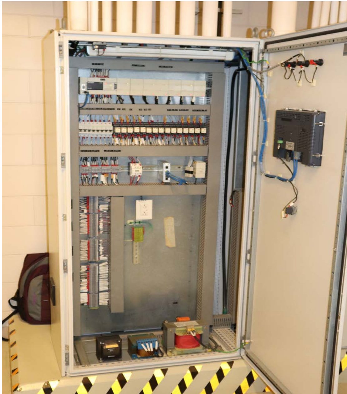
Figure 9 - Control Panel 2, Left Side, PLC, HMI, etc.
