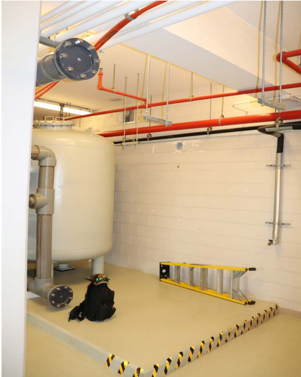
Figure 8 - Space for Pressure Filter 3
