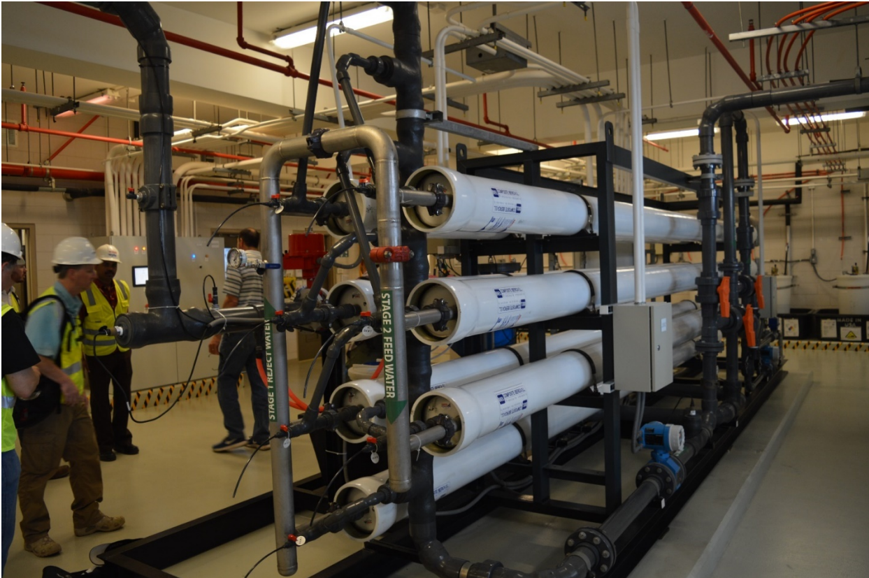
Figure 5 - RO Train 1 Rear Side
