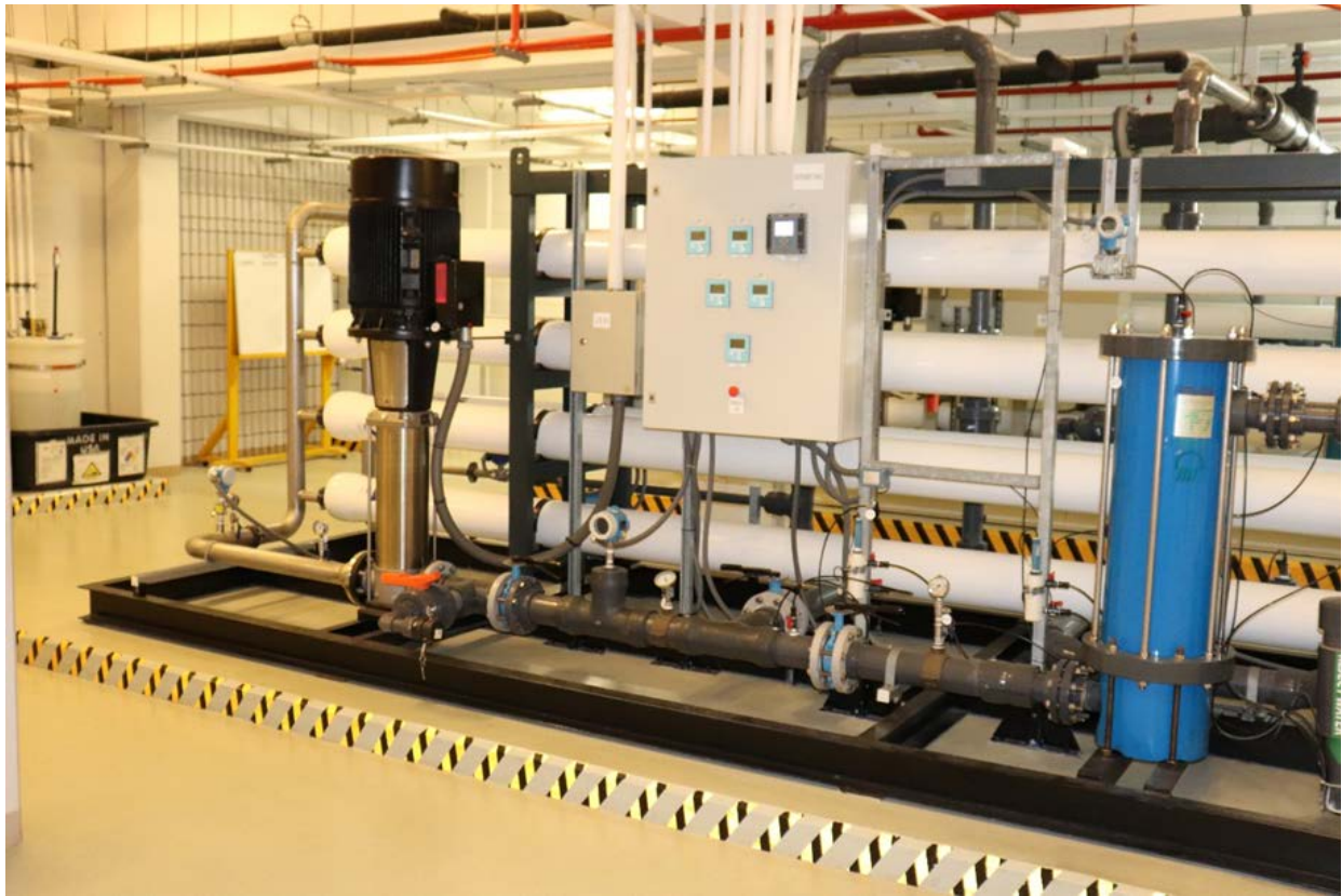
Figure 1 - RO Train 1, Left Front Side
