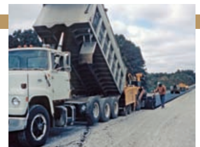
The Shelly Company paves Ohio's first rubblization project on I-70 in Muskingum County.
