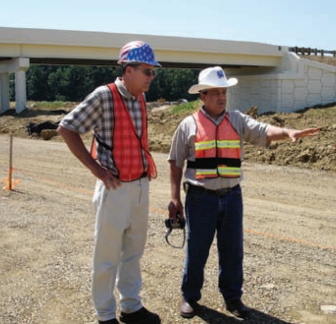
Fred Frecker and Ohio University researcher Shad Sargand survey the US 30 Test Road, developed to validate the design principles and extended life of the Perpetual Pavement.
