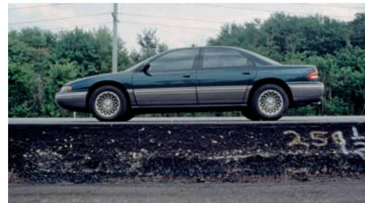
Armed with more and more research about its superior value, the industry aggressively promoted deep strength asphalt pavements.
