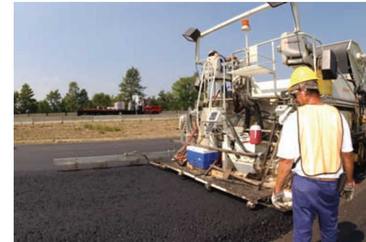
Northstar Asphalt places Ohio’s very first Perpetual Pavement on Stark County Interstate Route 77.
