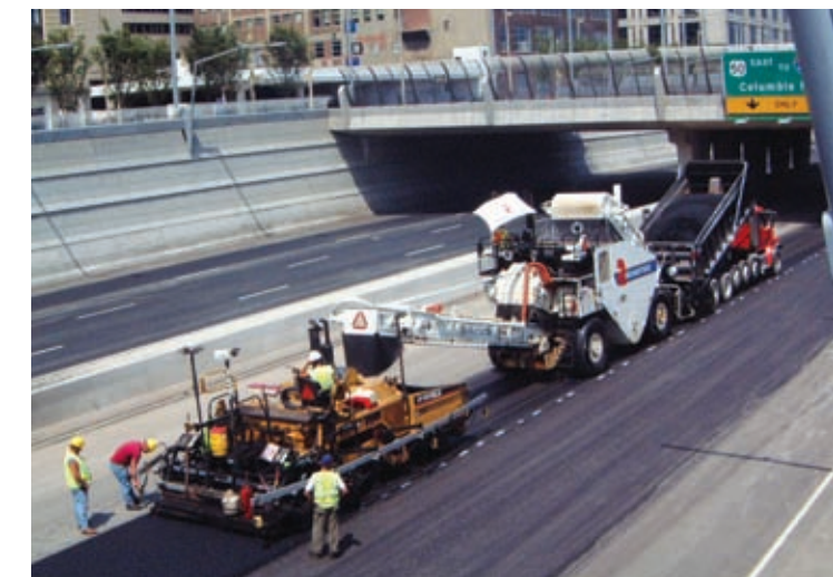
The reconstructed pavement for Fort Washington Way (I-71 and US 50) was one of the first applications of Stone Mastic Asphalt in Ohio.
