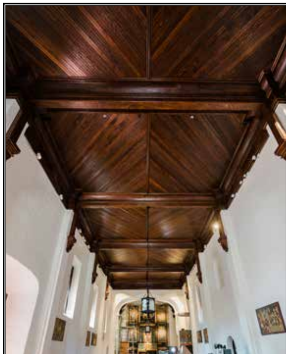
The mission's restoration team was so impressed by the color of the redwood beams in the mission's new ceiling that they decided not to paint over the wood. ( Simon Kim )
