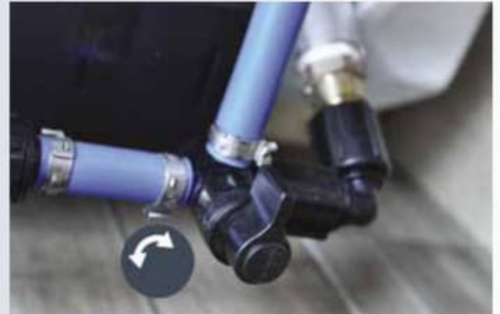
Water heater bypass & winterizing valves make draining the system for winter storage a breeze.
