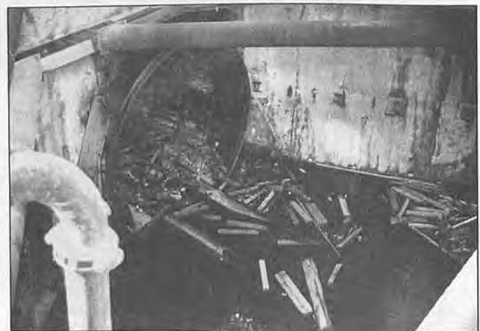
Burnt-out timbers and smoldering embers floated in the now-darkened water used earlier to put out the fire.
