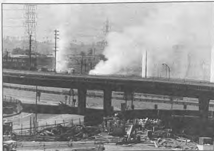
From a vantage point close to Macy Street and Vignes smoke is seen billowing from the cave-in across U.S. 101.
