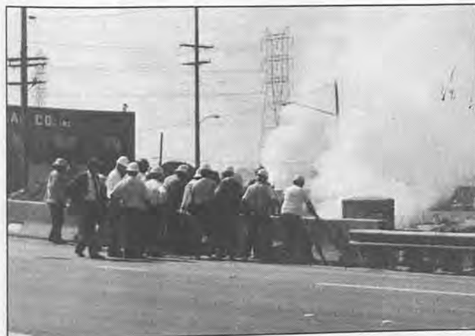
Metro Rail officials survey the damage caused by the fire and the subsequent cave-in from their perch on U.S. 101 which was closed down for four days.
