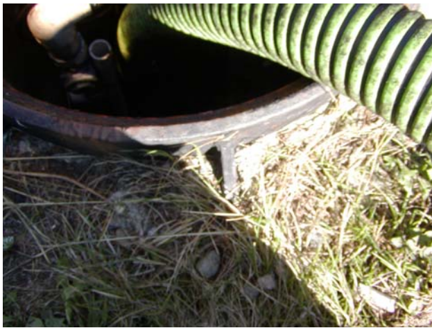
Minerva Beach - Laundromat and Pump Station
