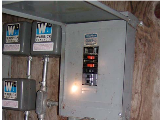
Minerva Electrical Circuit Breaker
