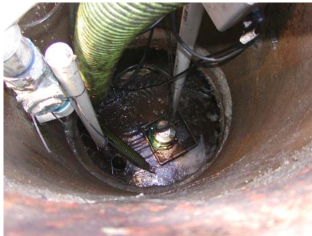
Minerva Beach - Laundromat and Pump Station
