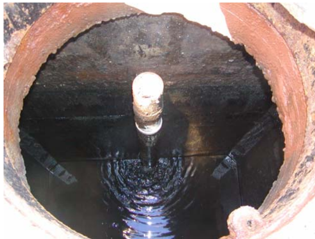
Potlatch State Park – Day Use Area Septic Tank
