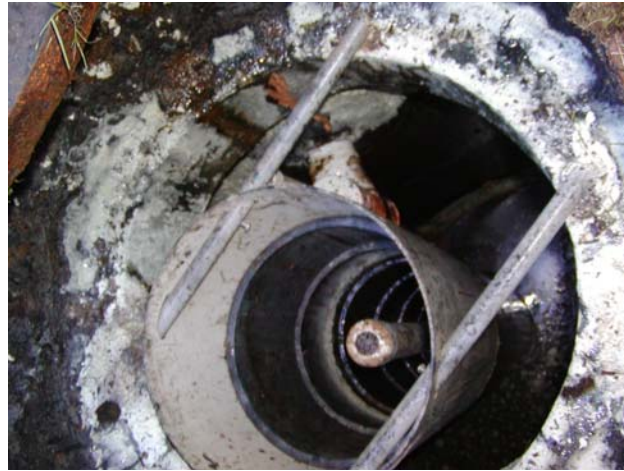
Potlatch State Park – RV Dump Septic Tank Bio-filter
