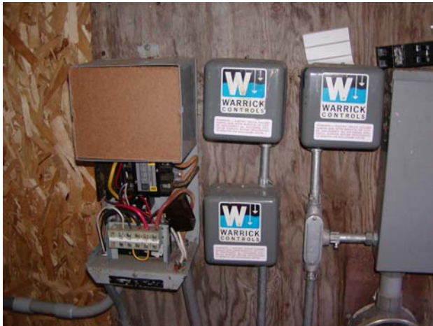
Minerva Well Controls
