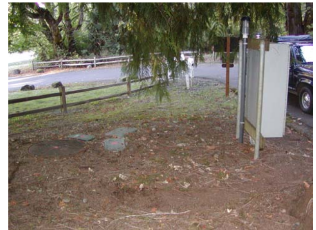
Potlatch State Park – RV Dump Station Control Panel
