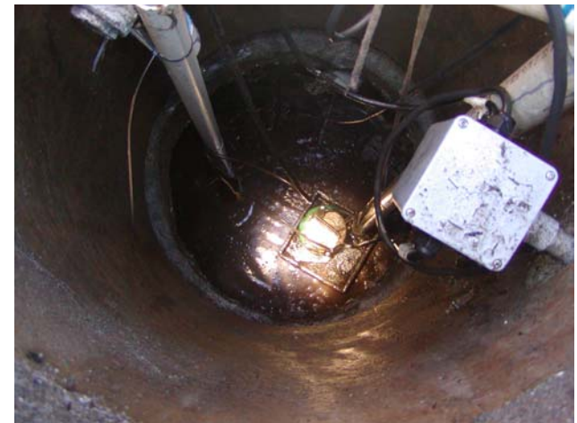
Minerva Beach - Laundromat and Pump Station
