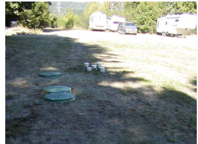
Minerva Beach - Drainfield Septic Tank
