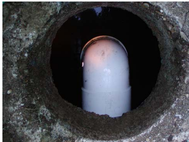
Minerva Beach - Drainfield Septic Tank
