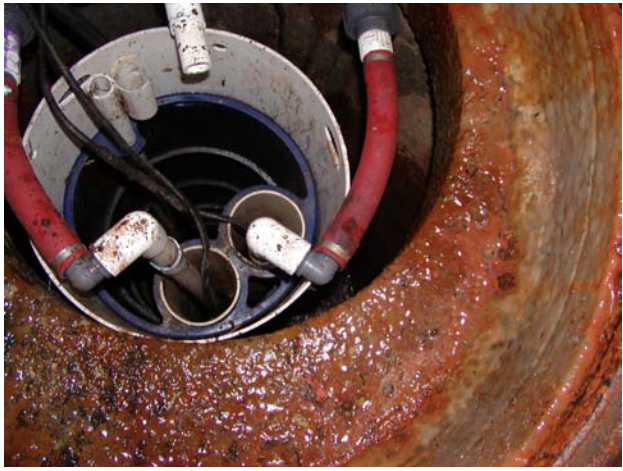
Potlatch State Park – RV Dump Pump Station
