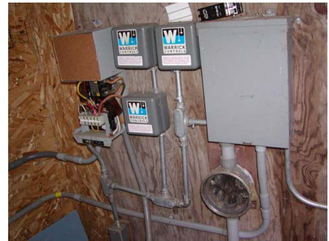
Minerva Well Controls
