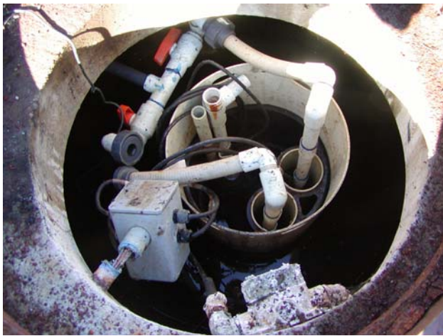
Potlatch State Park – Day Use Area Pump Station
