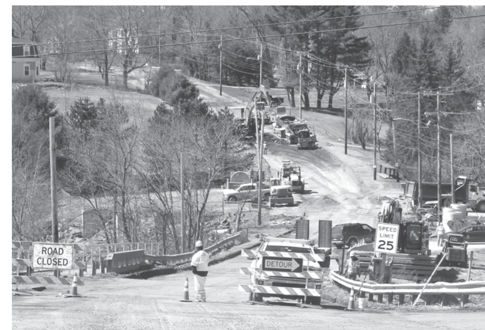
A crew works to remove the old Grist Mill Bridge in Hampden. The new "72-hour bridge," designed by Kenerson's son Tim, marks the completion of a Route 1A reconstruction that BACTS began more than 20 years ago.
