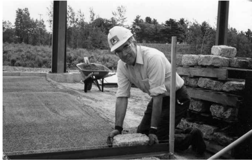
Galen setting the first cobblesone at the Cole Land Transportation Museum in 1998.
