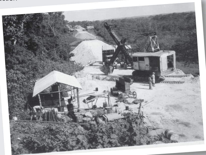
In a jungle clearing somewhere in México circa 1936, a P&H service crew changes out the track belts on a P&H shovel.
