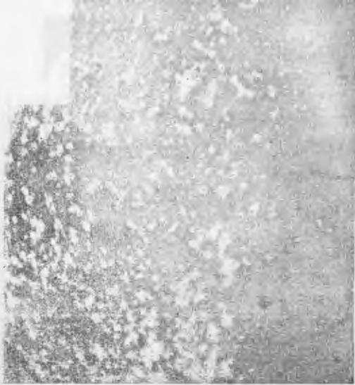
Rust Under Finish.
