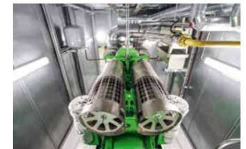
GENERATOR IN CHP PLANT
