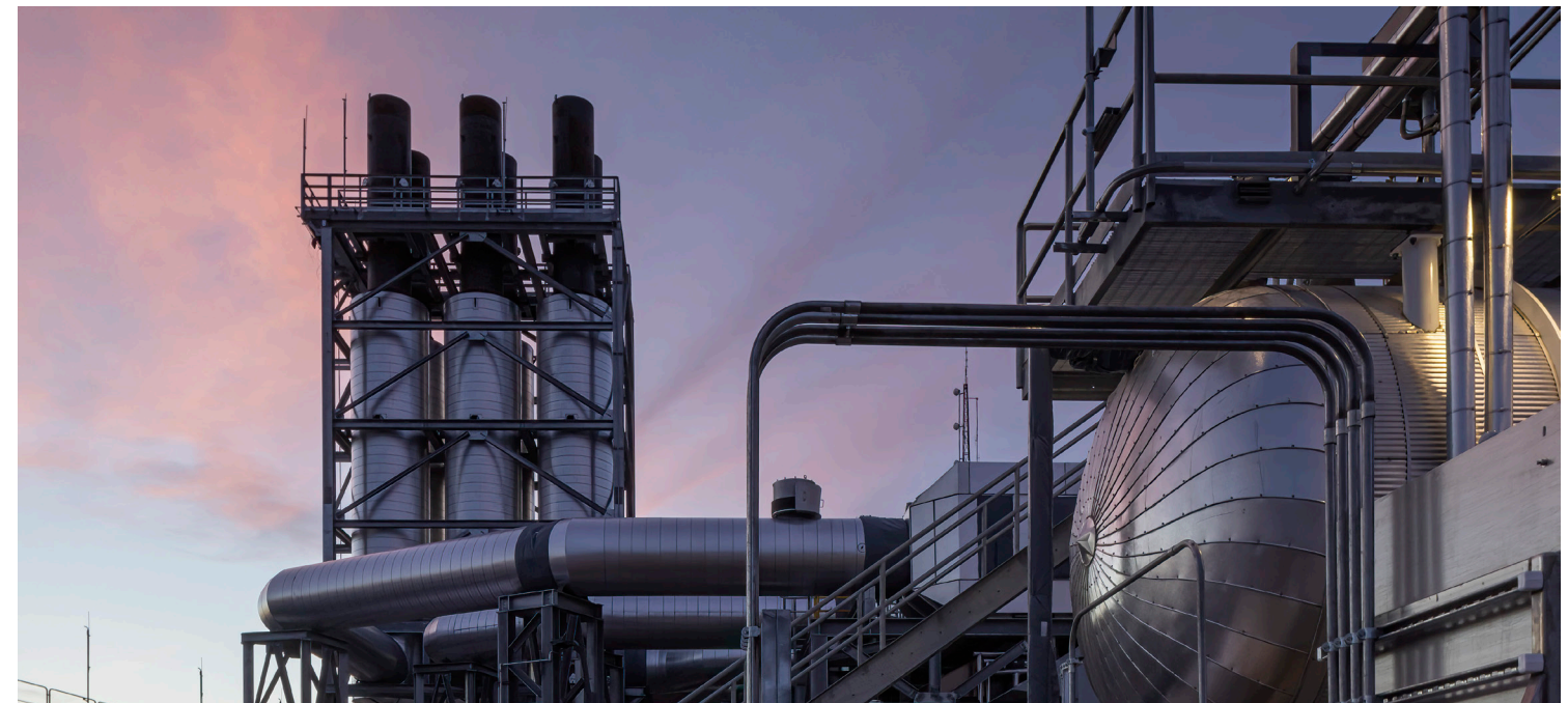
▲ Our 58-megawatt Bob Glanzer Generating Station in Huron, South Dakota, provides on demand resources to support the variability of wind and solar projects coming onto our system and helps serve our customers during extended periods of peak demand.
