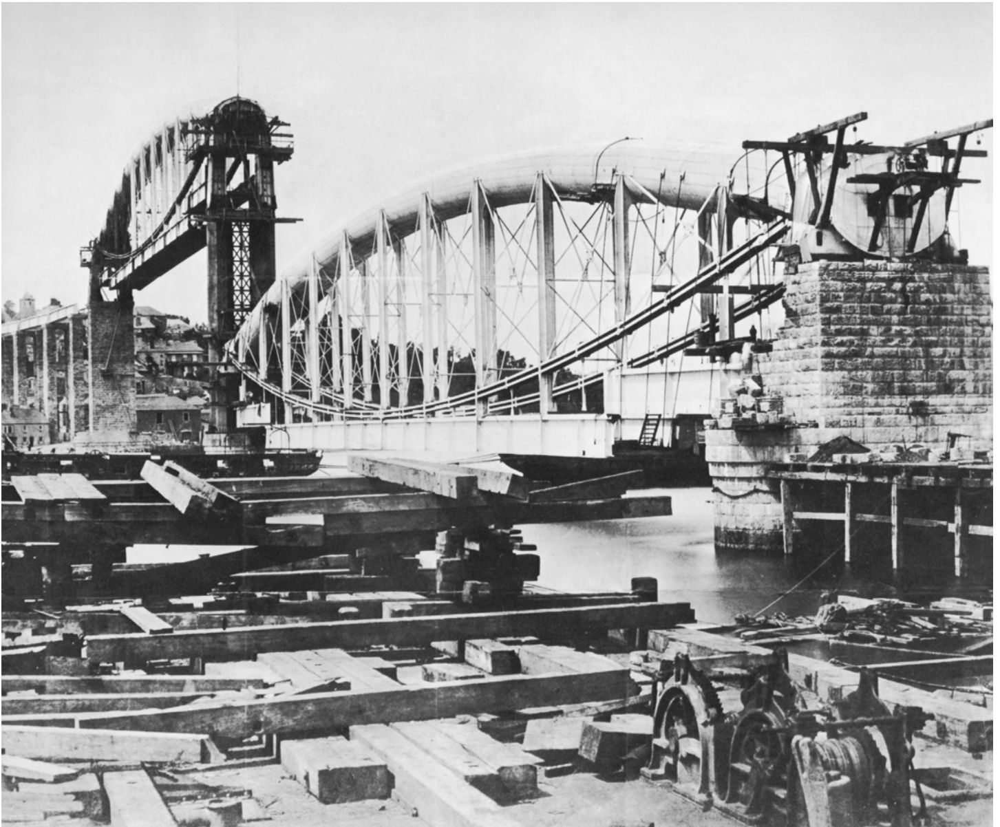
The Royal Albert Bridge, spanning the Tamar at the traditional crossing point from Plymouth to Saltash, under construction in the 1850s.
