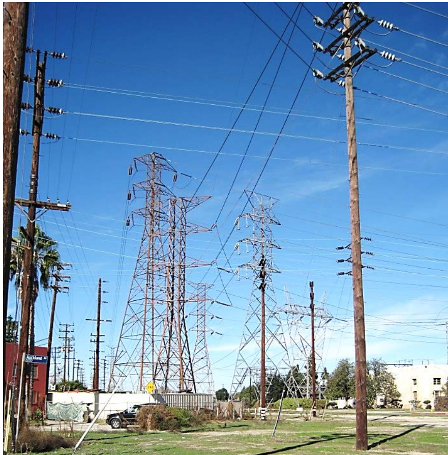
Transmission Line Towers
