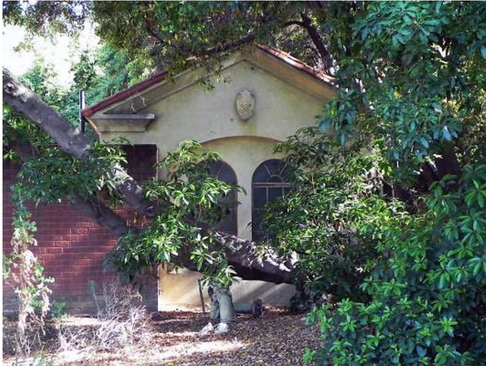
Laurel Canyon Pumping Station, circa 1930 and 1950 11300 Dona Dorotea Drive, Studio City (SurveyLA)
