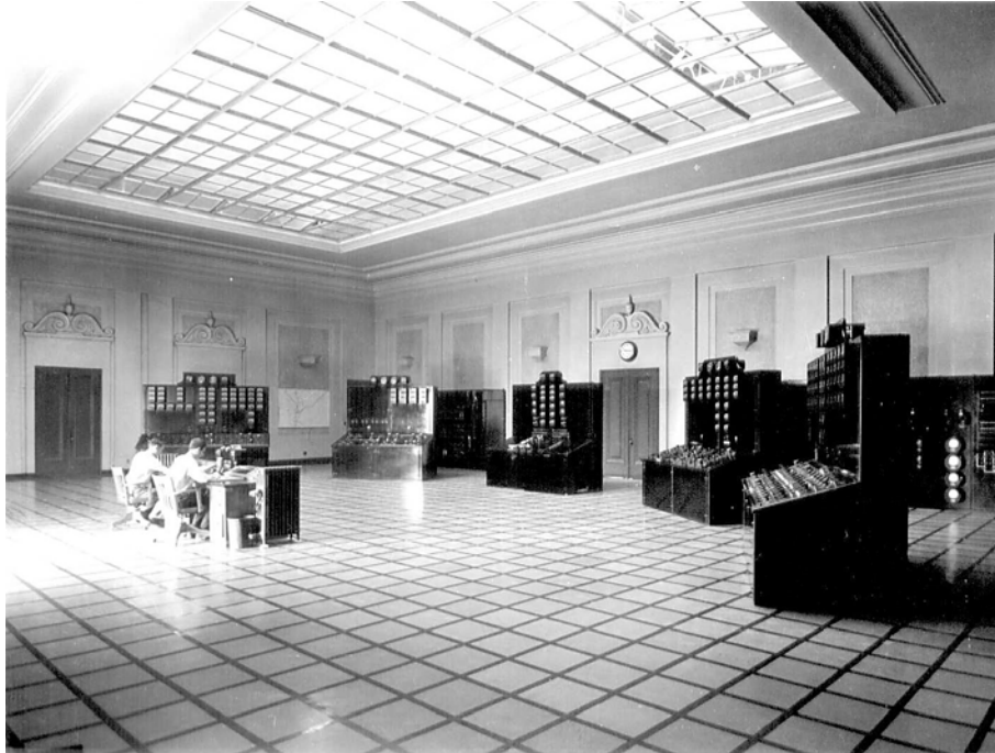
Control Room, Receiving Station B (Los Angeles Department of Power and Light)
