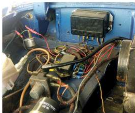
Electrical fault is hiding here – somewhere
