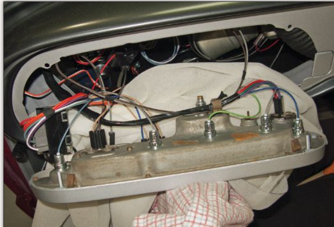
Though it never suffered from any animal invasion, the entire wiring harness had become brittle due to age and was completely replaced. The gauge cluster remained remarkably intact, with only a cleaning and a speedometer lube needed before re-installation.
