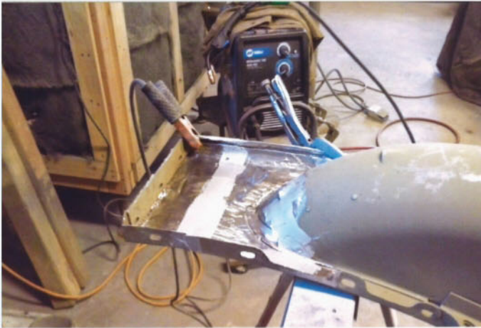
The main body and associated panels were also media blasted. Corrosion was restricted to two small areas, including the underside of the spare wheelwell within the front fender. Here, work continues on a patch panel that has been welded into place.
