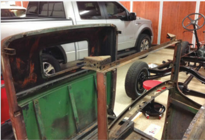
The remaining wooden roof structure appeared to be sound; however, after consulting knowledgeable Model A enthusiasts, it was recommended that all the wood within the cab be replaced with new pieces. Fortunately, dry rot had not affected the steel supports.
