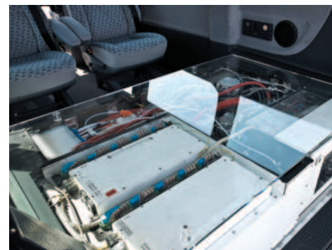
△ The technology reduced in size and now fitted in the floor.
