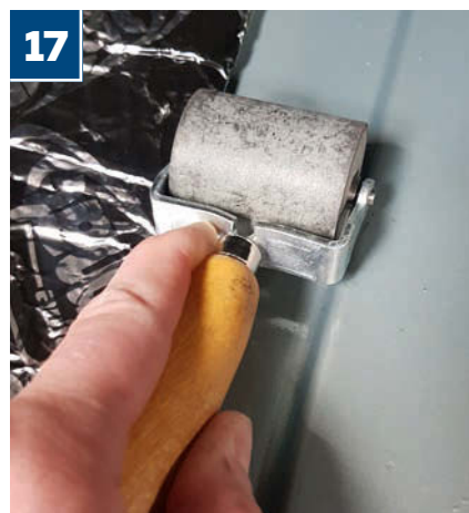
17 As you can see, the heavy duty roller available direct from Dynamat is the same width as the recess between each raised element of a Silver Shadow II's floor
