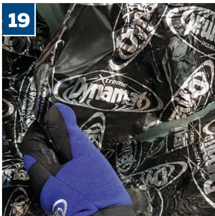
19 Don't be worried if the sheets you're working with crease on application, as using the roller will flatten them out; besides, curved and angled shapes, such as the rear suspension turrets, are unlikely to allow smooth fitment
