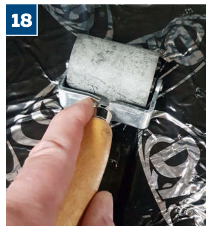
18 With the material carefully laid in place, you can start to work the roller into each crevice, though Dan recommends laying a sheet gradually, working the roller as you go
