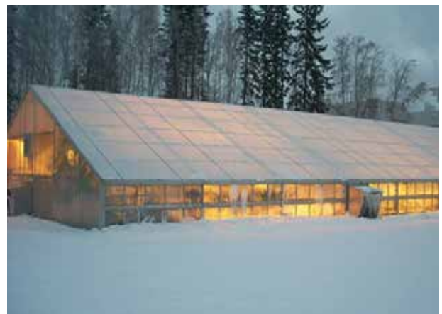
▲ A greenhouse stays warm during Wisconsin's cold winter thanks to a biomass boiler installation.
