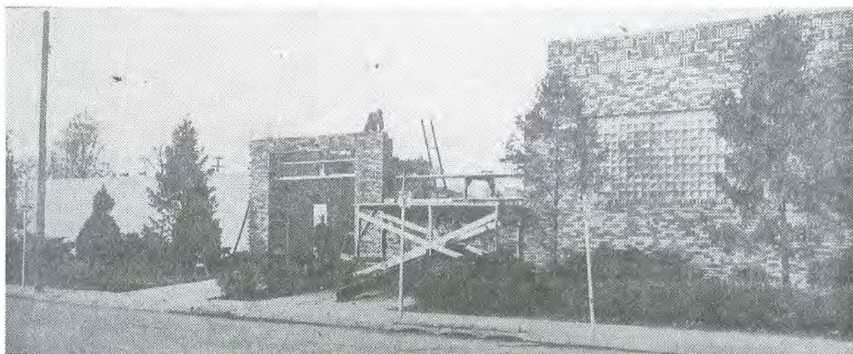
Figure 34. In December 1947, construction work on the new garage was well underway. View is to the NW. Source: Davenport Democrat and Leader , December 31, 1947.
