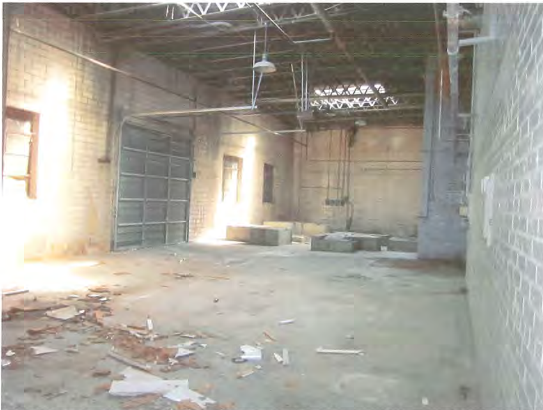
Figure 5. Part of the c.1950-52 Ice Cream Factory addition, Room D-3. Features the smokestack base (bump-out, center right), boiler room access (not shown, but further back on right-side wall on either side of smokestack base), glazed tile walls, two wired-glass skylights, and remnants of concrete machine platforms (toward rear of room). View is to NW Photo by Tallgrass Historians L.C., September 2010
