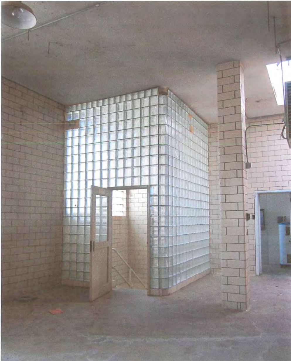
Figure 7. Glass-block-enclosed stairwell, Room D-4, Second Floor, Ice Cream Factory. This room also features glazed tile walls, service elevator access, and a wired-glass skylight (upper right). View to East. Photo by Tallgrass Historians L.C., July 2010
