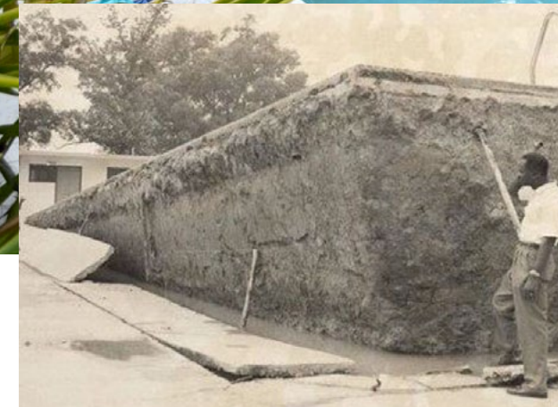
Swimming pool becomes buoyant during Hurricane Charley flooding. Photo appropriated from the internet.
