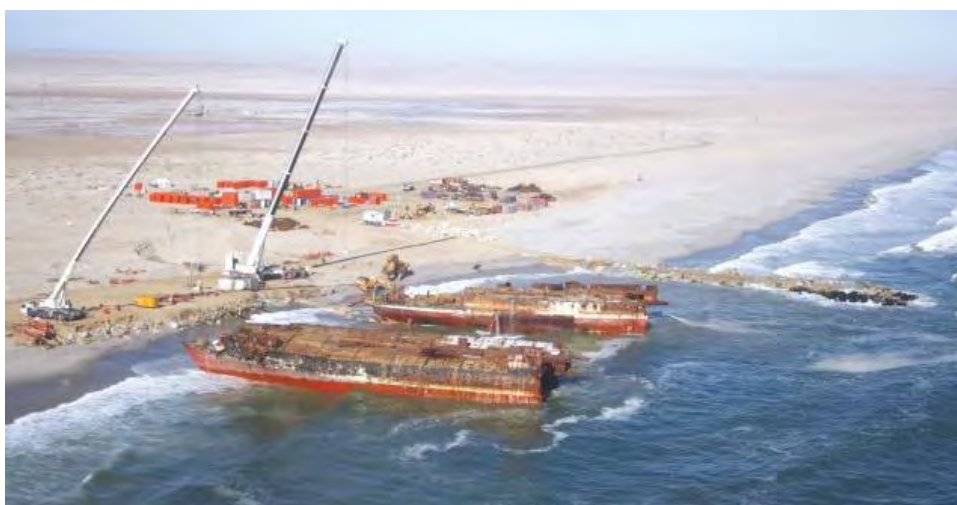
April 2013, to facilitate demolition the Chamarel was cut in two ©Allgemeine Zeitung-Namibia
