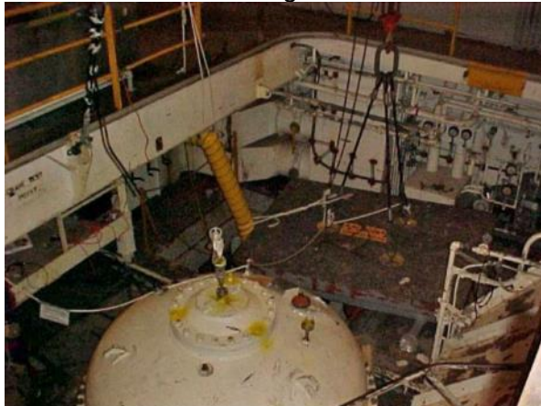
Refueling Room aboard Sturgis , showing Spent Fuel Tank Lid and Access Plug. (Corps Photo)
