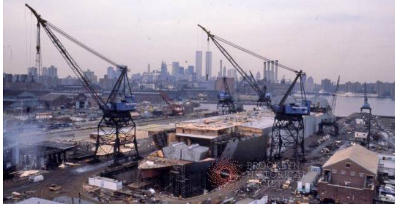
New York, 1978, Bay Ridge under construction © Frank J Trezza / Brooklyn Visual Heritage
