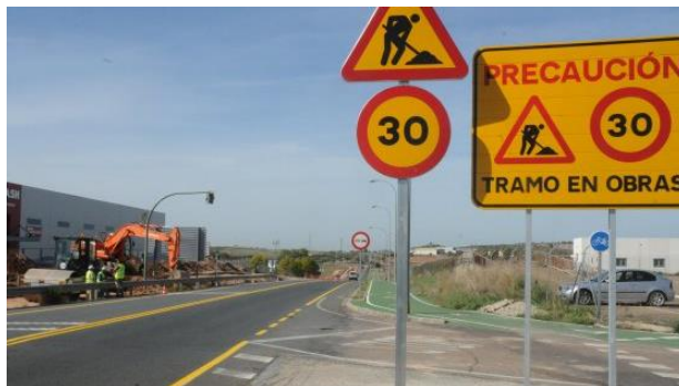
c. Temporary yellow pavement marking on a rural two-lane highway in Spain (circa 2013)
