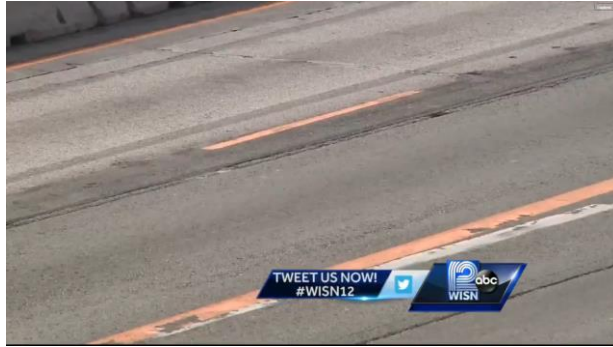
©2015 WISN-TV, Milwaukee, All Rights Reserved a. Zoo interchange orange markings in April 2015
