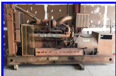
3 Each Allis Chalmers 475 KW GENSETS
