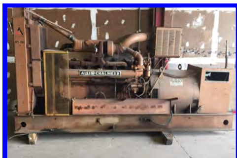
3 Each Allis Chalmers 475 KW GENSETS
