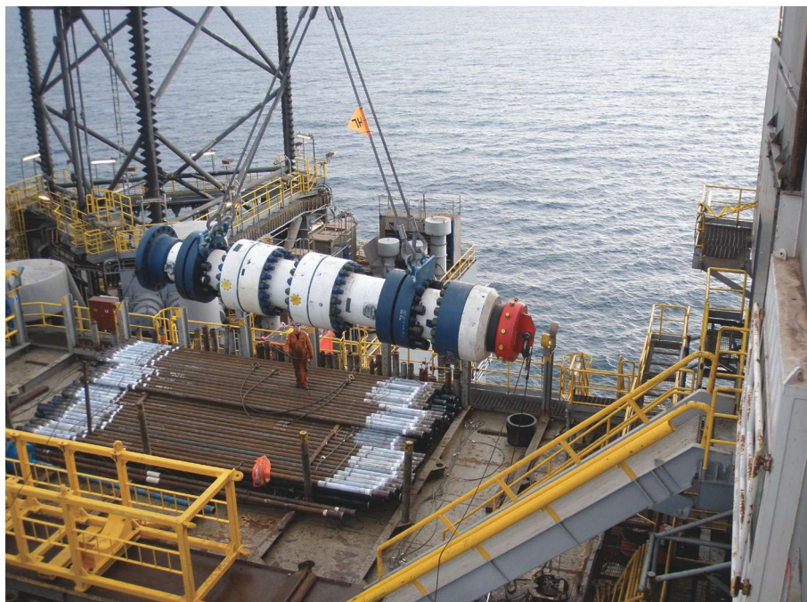
Plexus' POS-GRIP surface exploration wellhead was being prepared to be run through the rotary table and installed on the riser during recent operations in the North Sea. (Source: Plexus Holdings)
