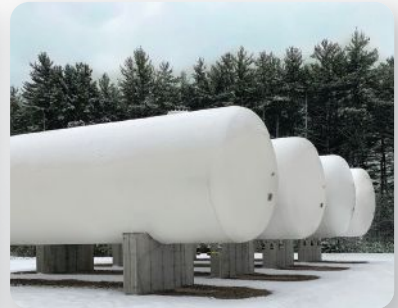
(3) 30,000 USWG, 250 PSI LPG Storage Vessel
