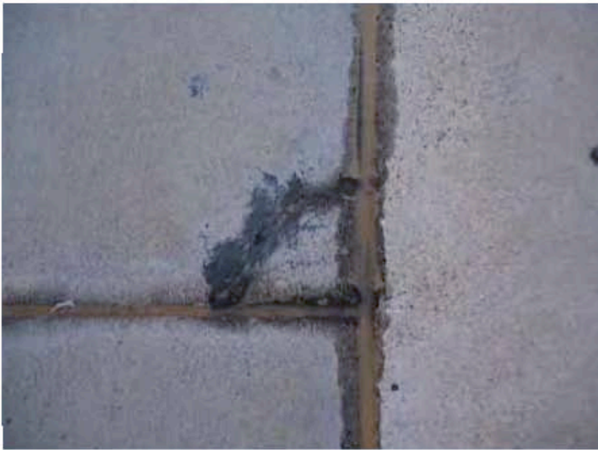
Photograph 29: Example of repaired pop-out on expansion joint corner.
