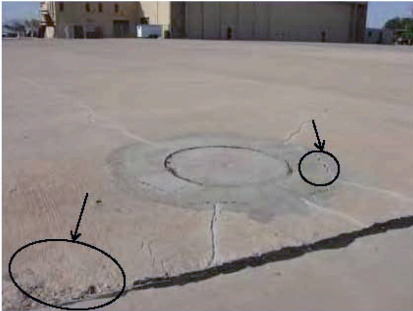
Photograph 11: A previous repair that may warrant additional repairs due to additional cracking and the presence of spalling. Most of the previous repairs within this area are still intact.
