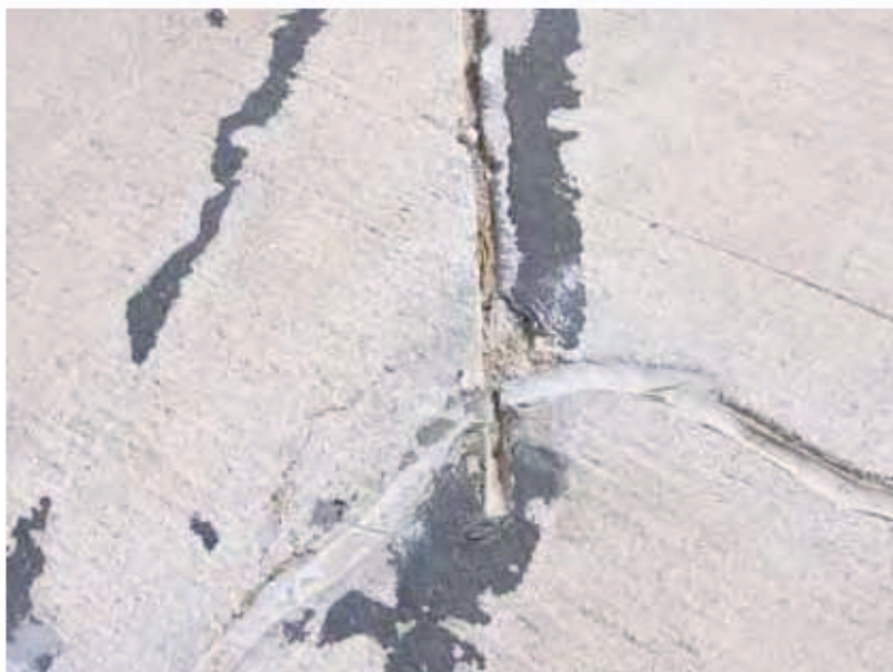
Photograph 9: A previous repair that may warrant additional repairs due to additional cracking and spalling present adjacent to the repair.
