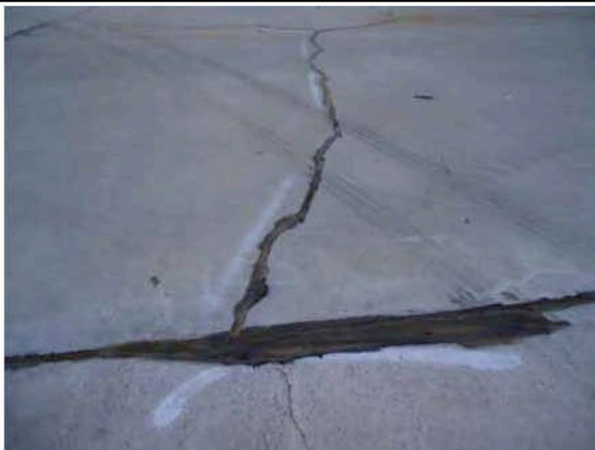
Photograph 22: From 2011 inspection, example of concrete crack that has been repaired (December 2010) and is in good condition.
