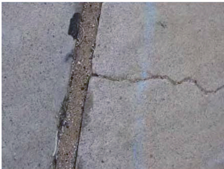
Photograph 15: Hairline concrete fracture intersecting with expansion joint.
