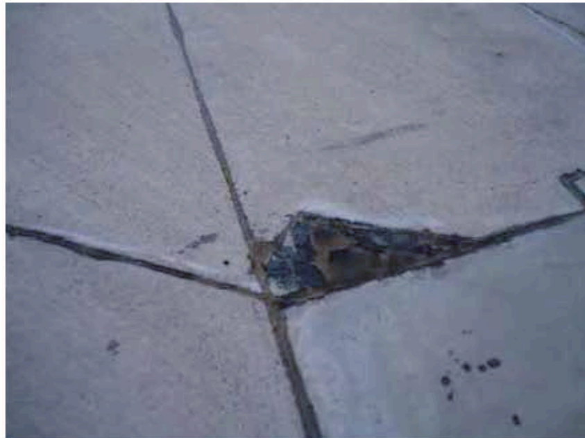
Photograph 23: Repair sealant in corner where spalling had been previously observed.
