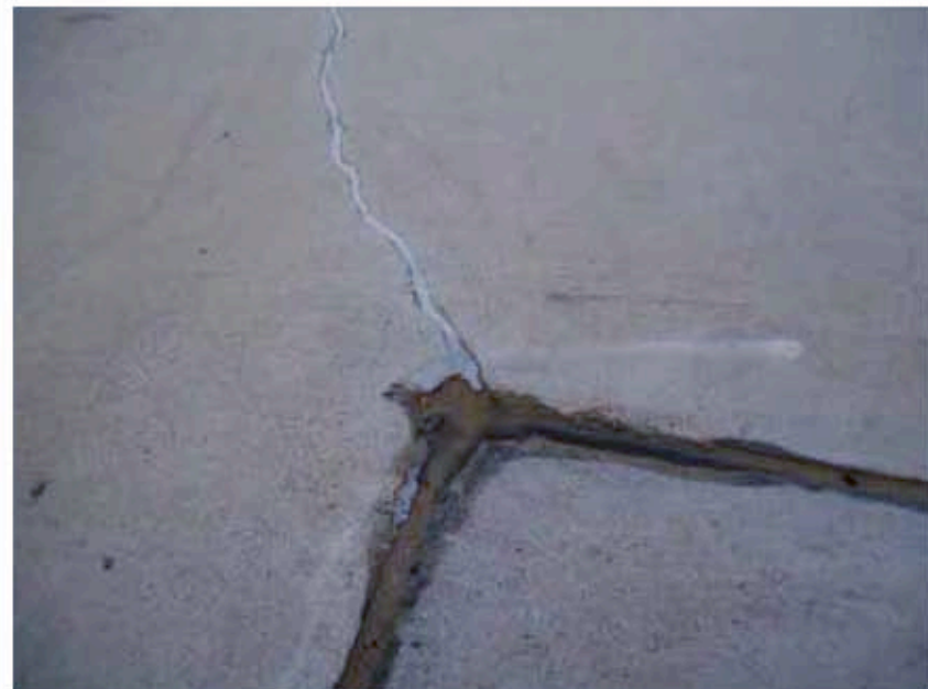
Photograph 24: Example of several generations of repairs.
