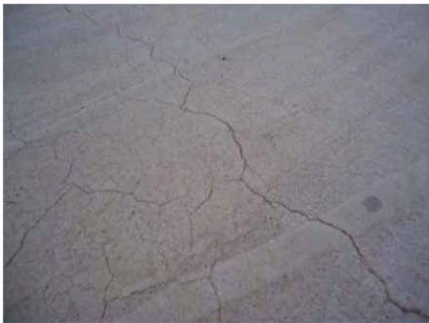
Photograph 25: Hairline cracks that will continue to be monitored.
