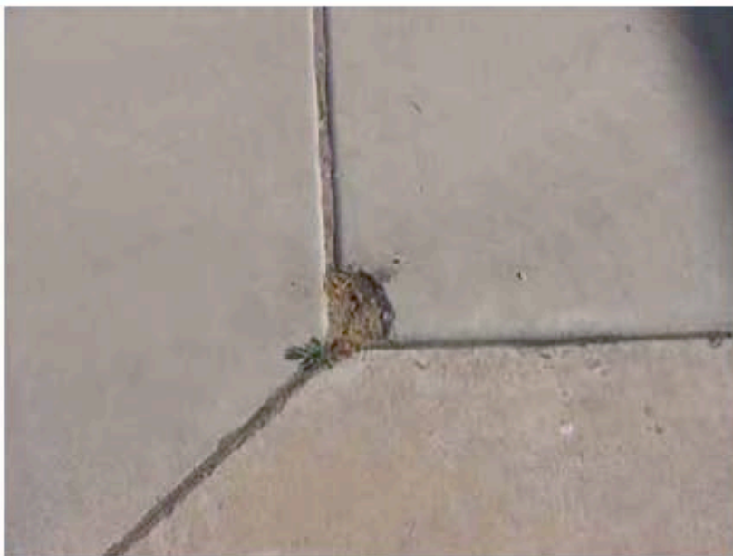
Photograph 12: A location in which a concrete popout has occurred at a corner joint. Repair may be warranted.
