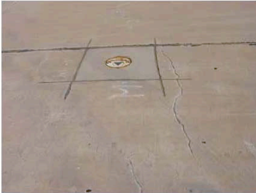
Photograph 2: January 2009 repair of concrete cuts around well completion, repairs performed by Tierra Dynamic.
