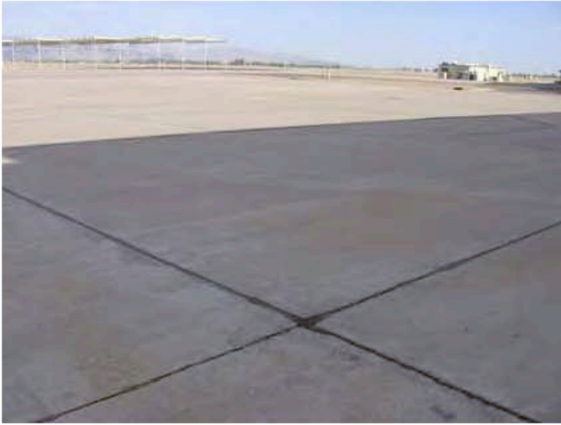
Photograph 1: Start of one of the transects walked during the 2009 cap inspection, standing next to Building 993 looking west across the cap.
