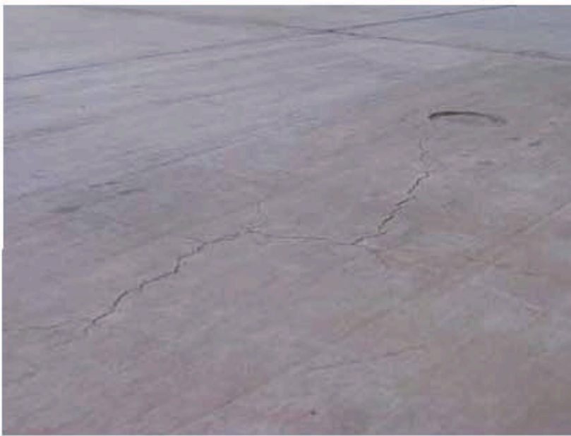
Photograph 8: Example of shallow surface cracking. Cracking with vertical or horizontal displacement are considered to penetrate the full depth of the concrete thickness.
