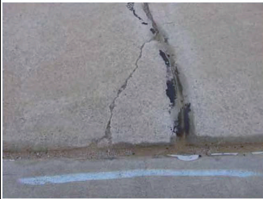
Photograph 19: Earlier repair that may warrant additional work due to presence of spalling and missing repair material.
