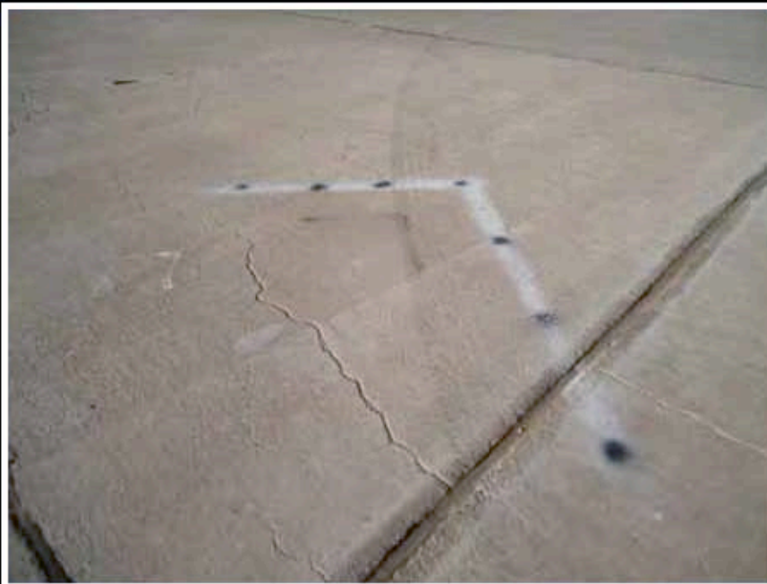
Photograph 31: Example of small crack at corner of concrete cap area.
