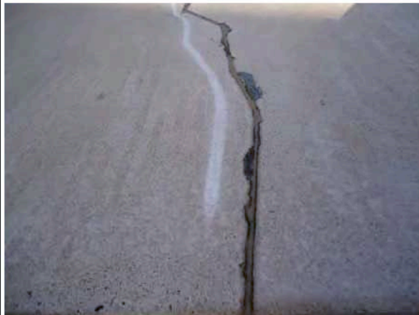
Photograph 32: Example of repaired crack that had limited spalling.
