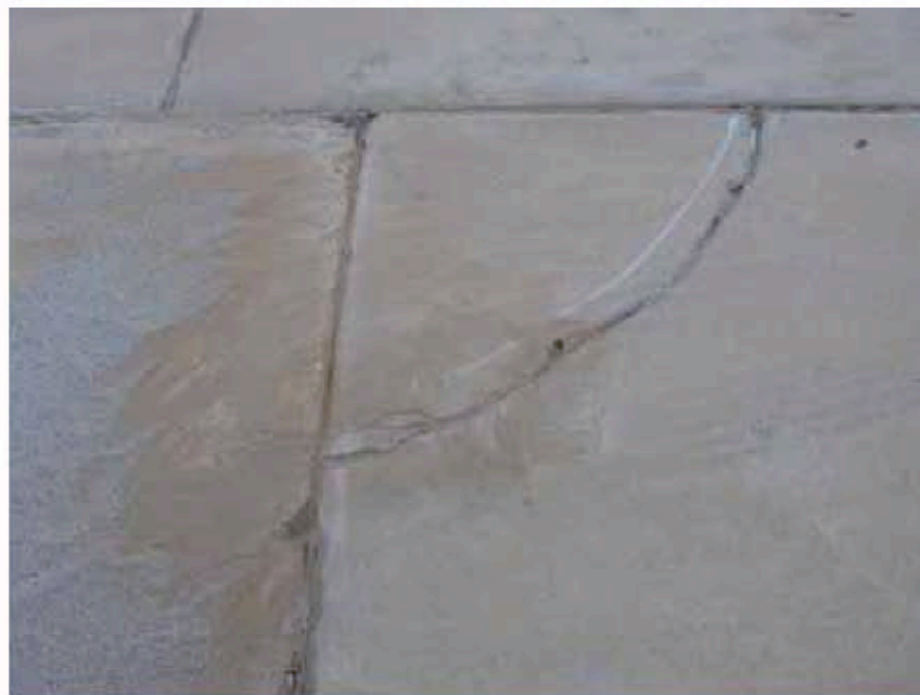
Photograph 14: Concrete crack that may warrant additional repair work; spalling observed adjacent to the crack and some gaping of repair sealant.
