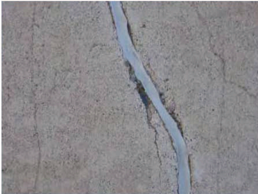
Photograph 17: Example of spalling adjacent to previous crack repair.
