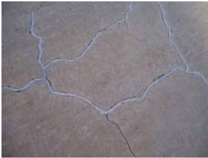
Photograph 28: Hairline crack coming off of previously repaired cracks; area will continue to be monitored.
