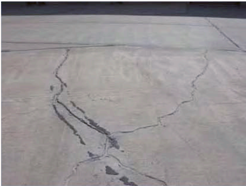
Photograph 7: A previous repair that may warrant additional repairs due to additional cracking and lack of repair material within the repair.
