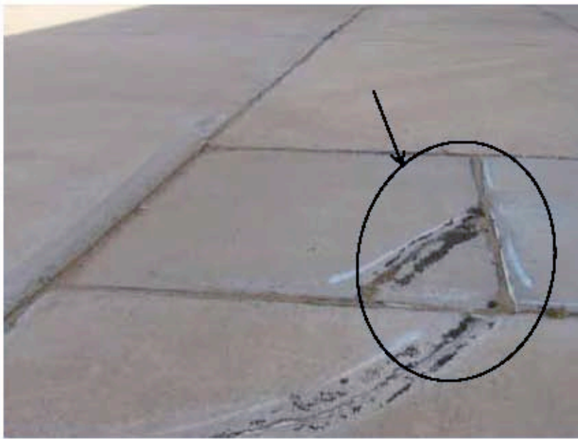
Photograph 10: A previous repair, that may warrant additional repairs due to additional cracking, the presence of spalling, and lack of repair material within the repair.
