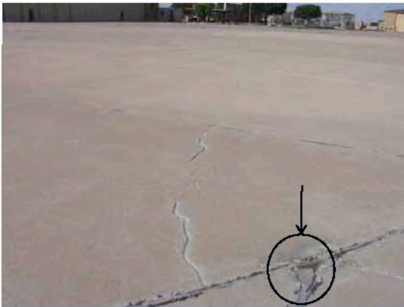
Photograph 5: A previous repair that may warrant additional repairs due to additional cracking and spalling present adjacent to the repair.
