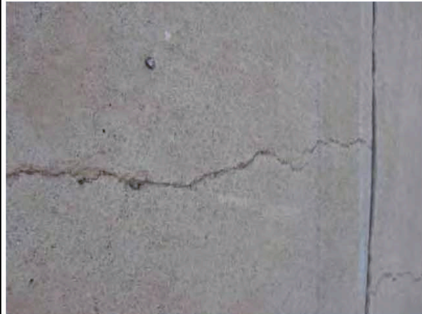
Photograph 20: Concrete crack, intersecting expansion joint, that is several feet long.
