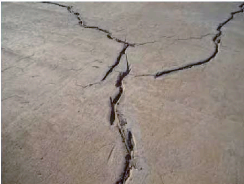
Photograph 30: Example of cracks that have been saw cut and repaired.
