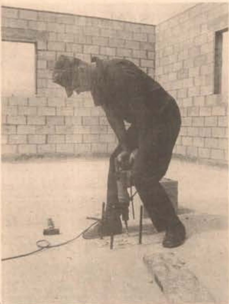
FROM THE GROUND UP — Corporal Wayne Winter, Facilities Support Self-Help, drills a re-bar setting for a concrete footing in the new Security Medical Storage Building. The building is scheduled to be completed by the end of the month. (Photo by SSgt W.S. Saunders)
